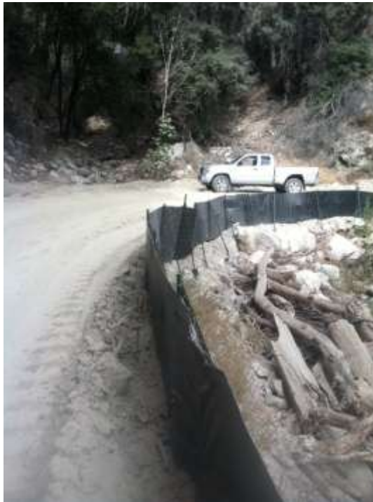
Figure 2: JD ID 6-67-S-4 is shown to have sediment, from access road construction, blocking the drainage on Segment 6 Loop Road L.
