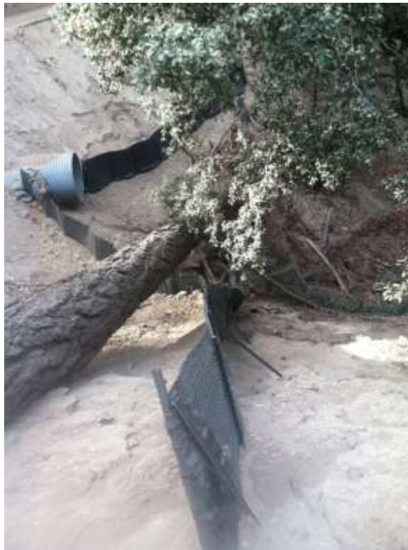
Figure 3: JD ID 6-68-S-62 on Segment 6 Loop Road L is shown with a downed tree covering/ crushed the perimeter silt fence of the culvert outlet and lack of mid slope BMP installed.
