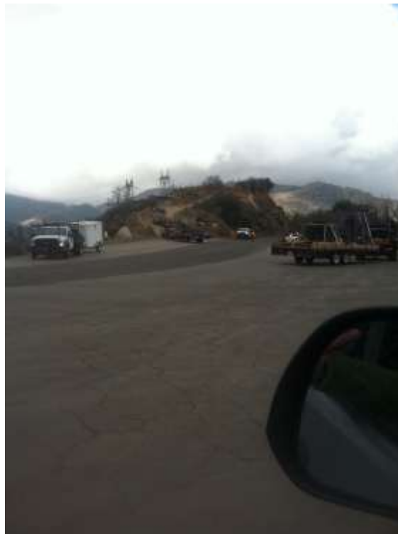
Figure 2: Wire trucks mobilizing onto Loop Road L for wire activities on Segment 6C.
