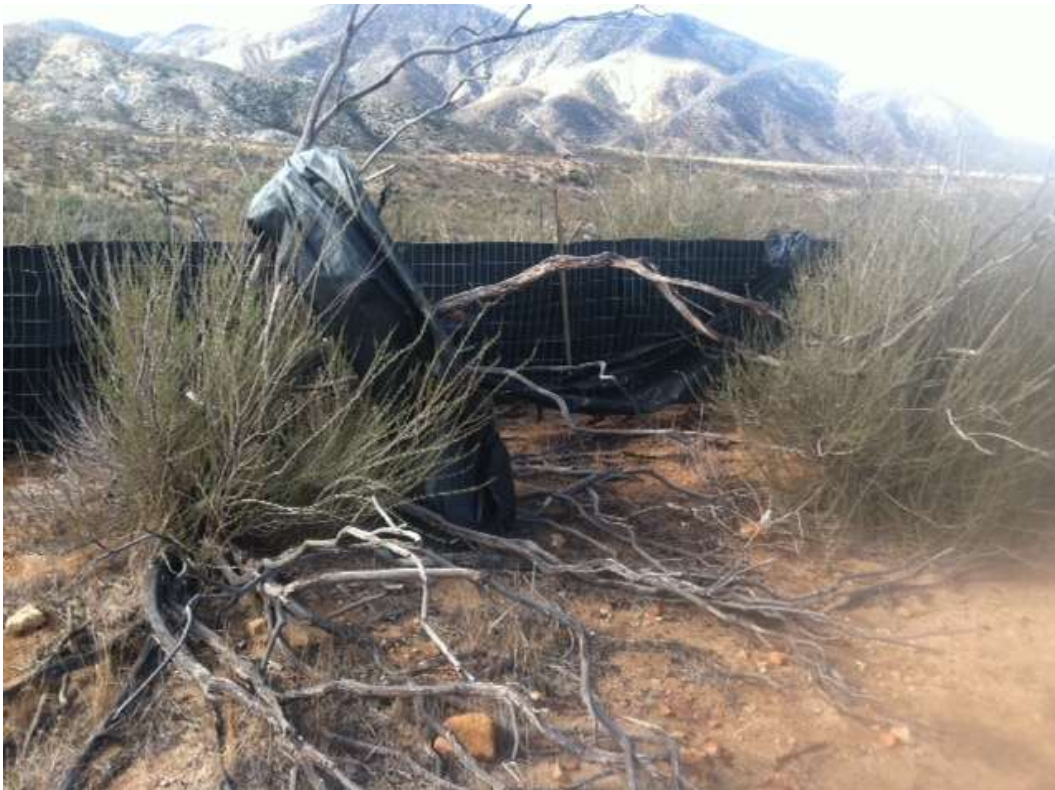
Figure 4: Unsecured silt fence at the Aliso HAY on Segment 6.
