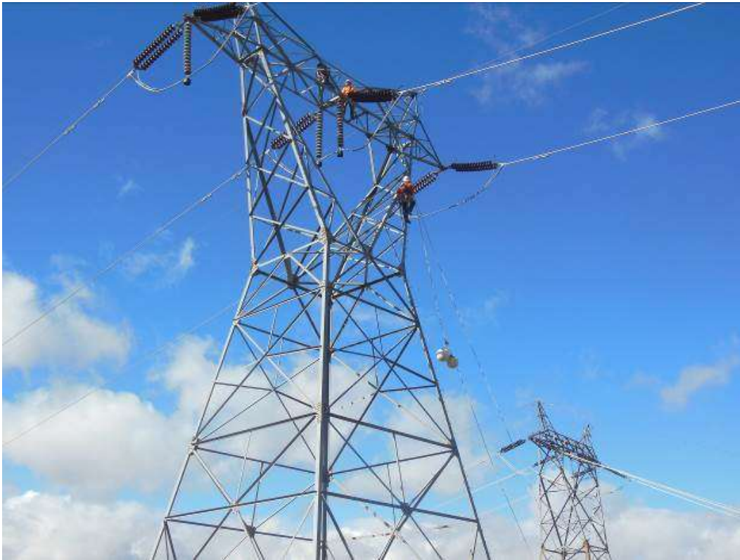
Figure 3. PAR crews installing bird nest deterrent buoys within the Pardee Junction area (between Constructs 13 and 19).
