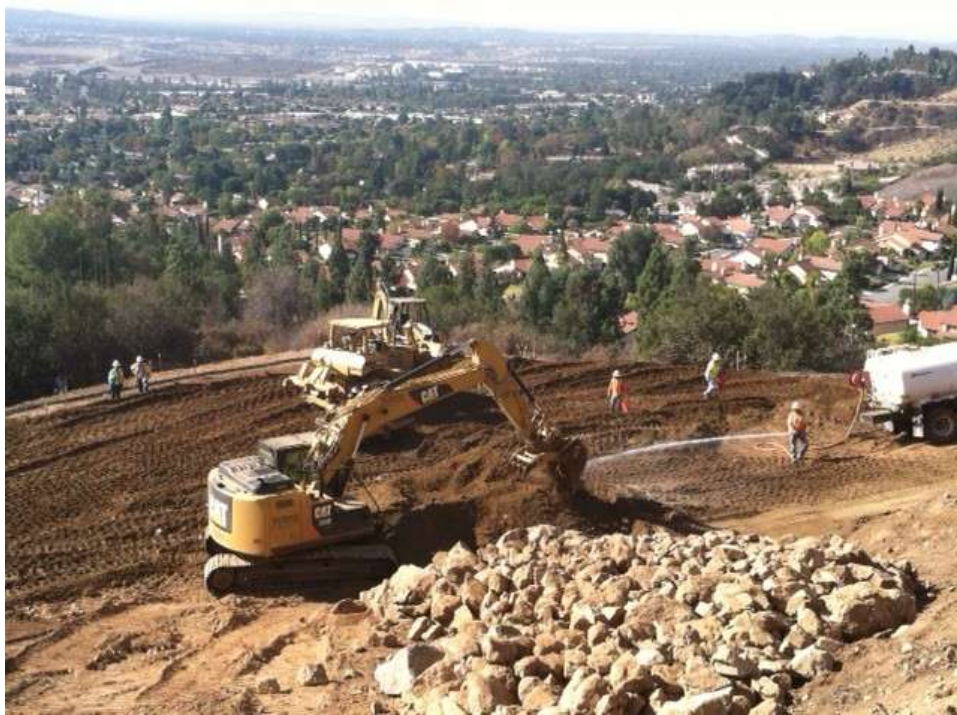
Figure 5: Union Engineering crews grading access road to Tower M27-T3 in Duarte, Segment 7.
