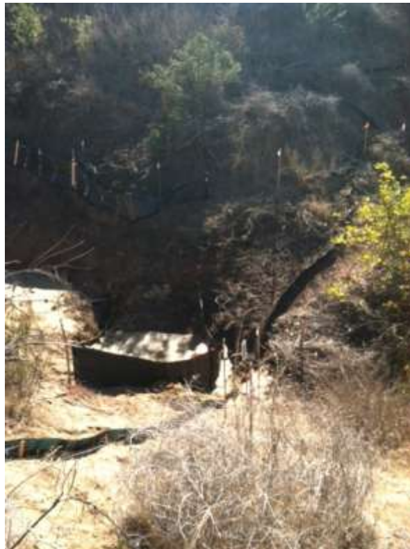
Figure 8: Sediment and water overflow of BMPs after accidental water release at Tower M57-T1, Segment 8.
