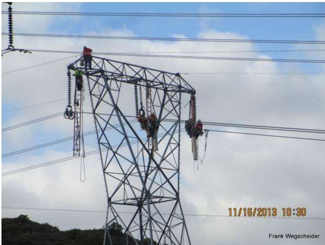
Figure 6: Installing travelers for wreck-out of existing wire between Constructs 2 and 11, Segment 11 (photo courtesy of FRED).
