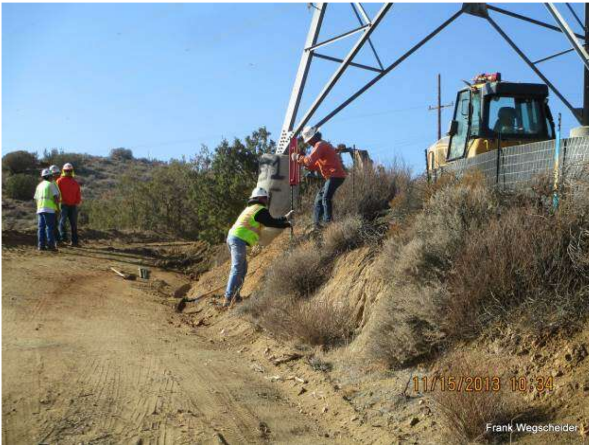
Figure 3: Installation of silt fencing BMPs at Construct 5, Segment 11 (photo courtesy of FRED).
