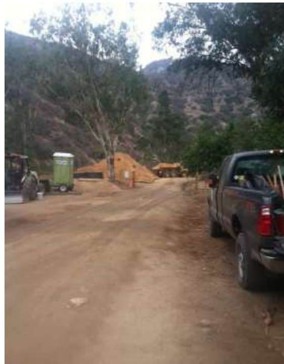
Figure 2: Dirt hauling from Construct 113 on Segment 6 to the Van Tassel Horse Ranch for hauling offsite.
