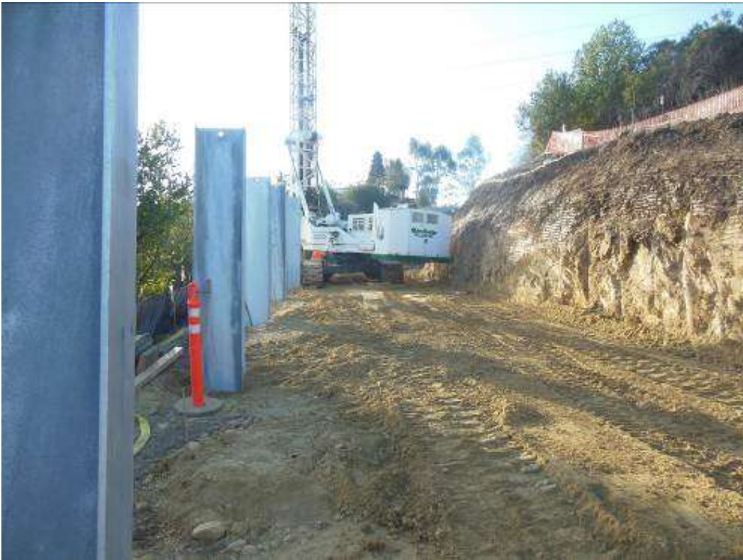
Figure 7: Western Foundations installing foundations for soldier wall at Tower M49-T1, Segment 8, Phase 4.
