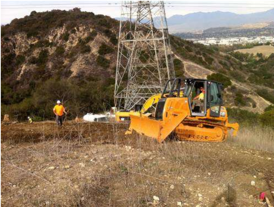
Figure 5: Warren James crews road grading at Tower M50-T4, Segment 8, Phase 4. (Photo courtesy of FRED.)
