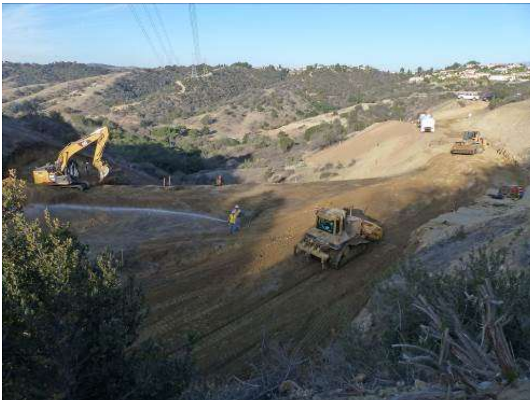
Figure 4: Union Construction conducting grading activities at Tower M57-T1, Segment 8, Phase 1. (Photo courtesy of FRED.)
