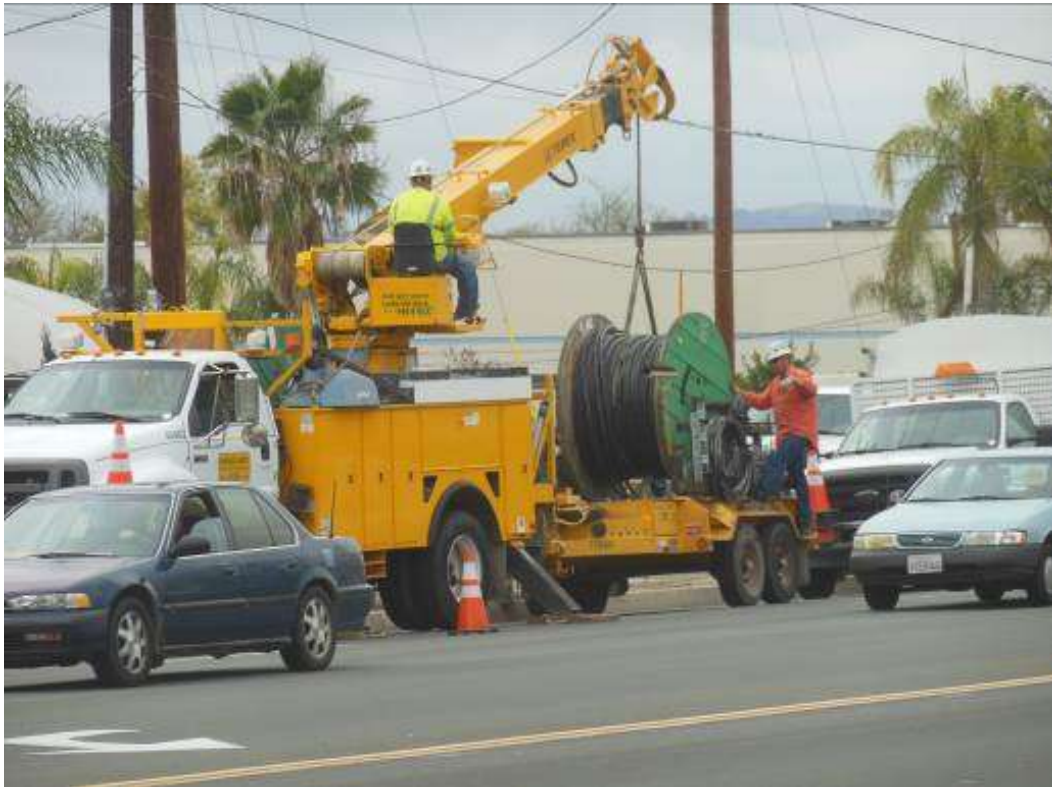
Figure 5: Preparing for wire pull through vaults at intersection of Edison and Central Avenues.
