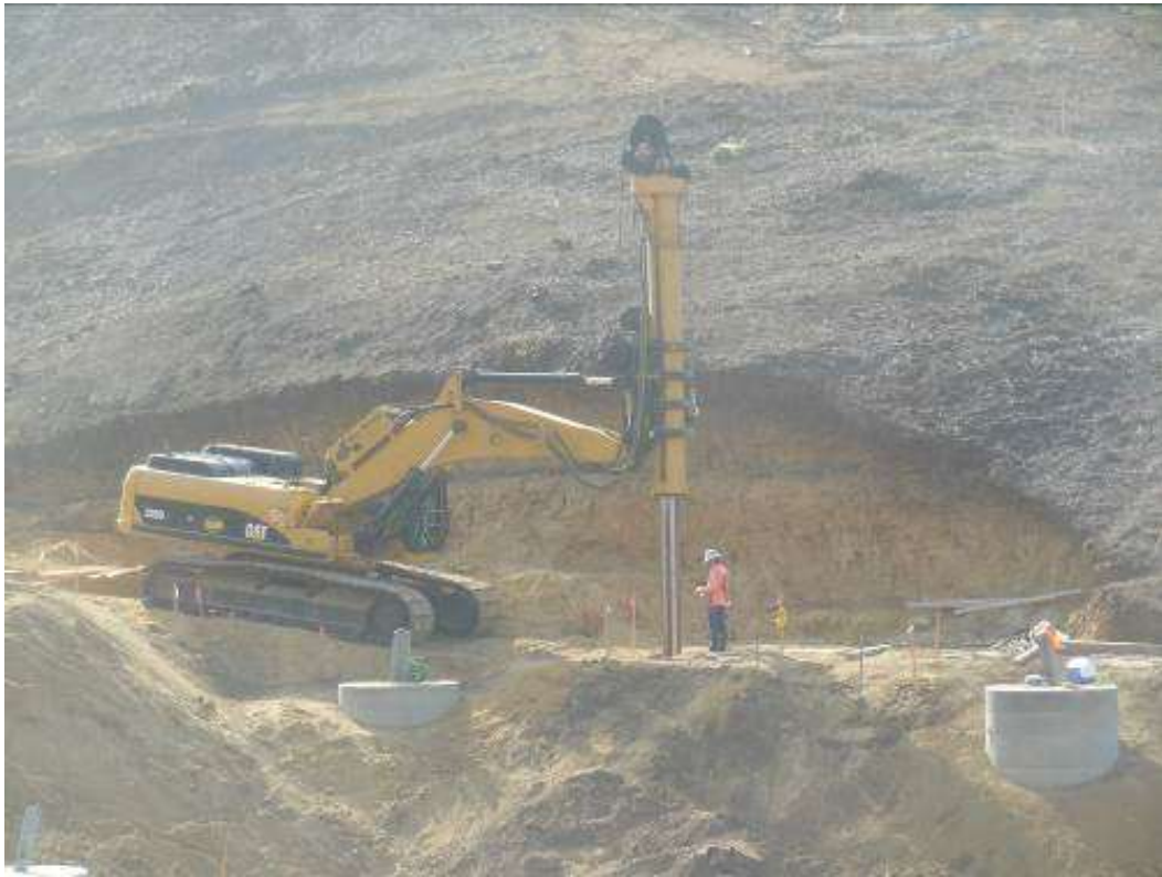
Figure 7: Drilling foundation holes for retaining wall installation at Tower M57-T1, Segment 8, Phase 1.
