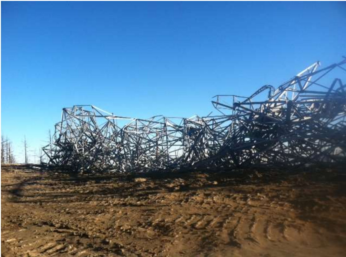
Figure 3: Structures removed from Segment 11C by the Skycrane were stored at Camp 16 for disposal.
