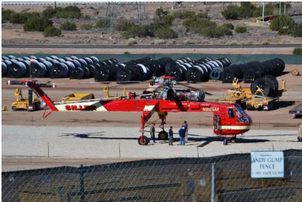
Figure 2: Skycrane helicopter used to remove old towers on Segment 11C, ANF lands.
