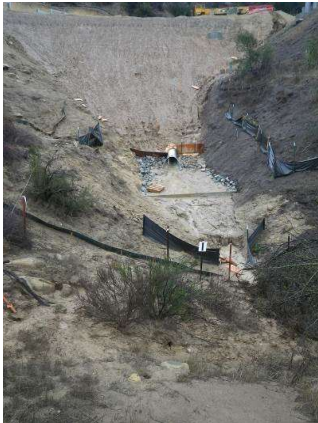
Figure 8: BMPs (silt fence and sandbags) blown out due to storm flows at Tower M57-T1, Segment 8, Phase 1 (photo courtesy of FRED).
