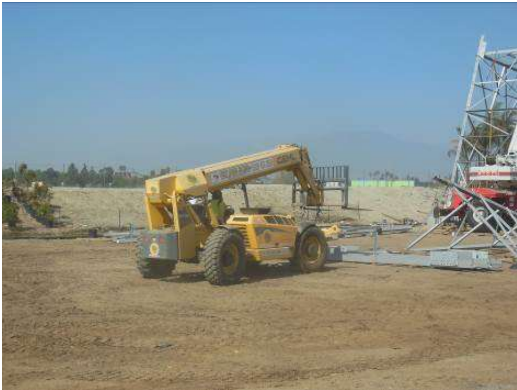
Figure 10: Forklift driving outside of approved disturbance limits (blue staking) at Tower M35-T3, Segment 7
