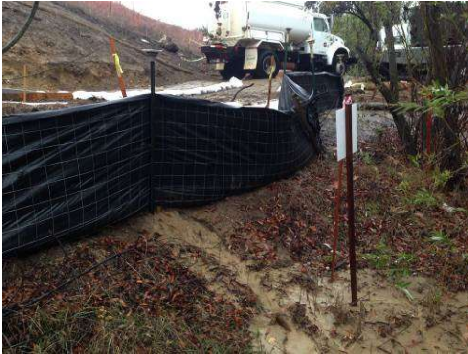
Figure 7: Runoff breaching silt fence BMP at Tower M49-T1 and flowing into JD ID# ID# 8-20-S-400, Segment 8, Phase 1 (photo courtesy of FRED).
