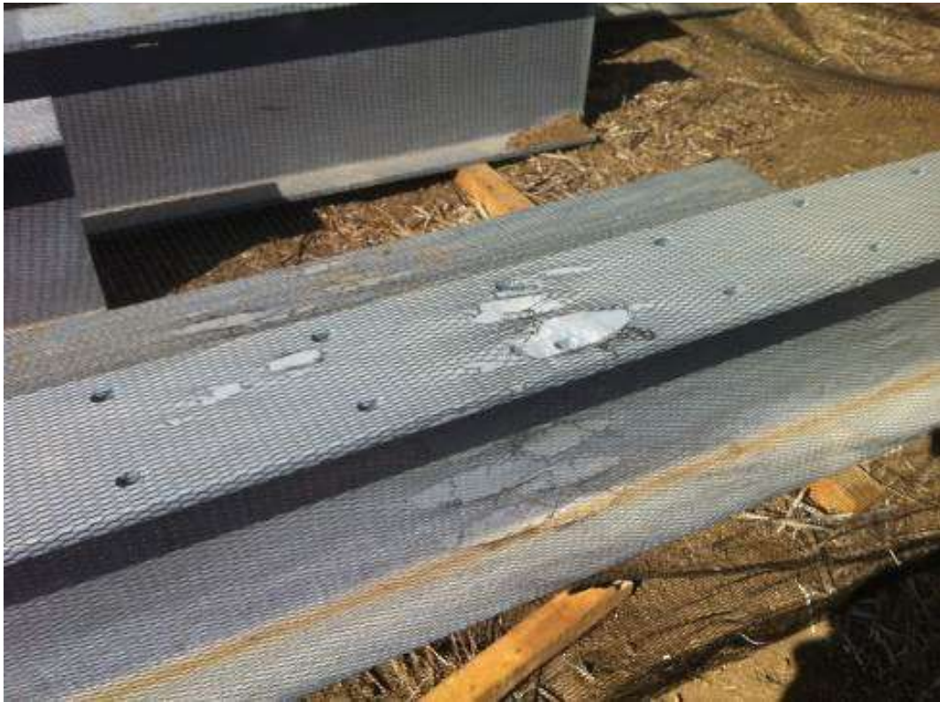
Figure 9: Holes in bird netting observed near Tower M57-T2, Segment 8, Phase 1 (photo courtesy of FRED).
