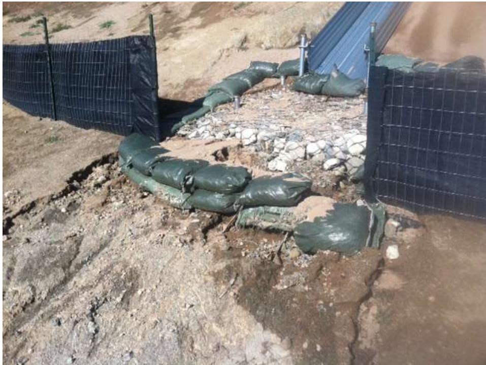
Figure 3: Sediment filled rock dissipater at Construct 5, Segment 6A.
