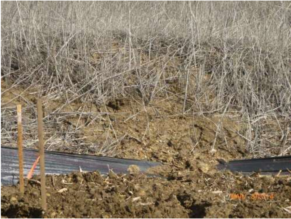
Figure 9: Post storm inspections identified multiple locations where sediment overtook BMPs and traveled off site, including Tower M49-T1 (photo courtesy of FRED).
