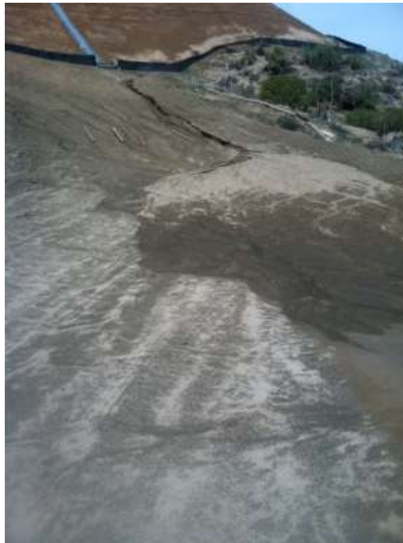
Figure 5: Gullying seen on the slope beyond Construct 5, Segment 6A.
