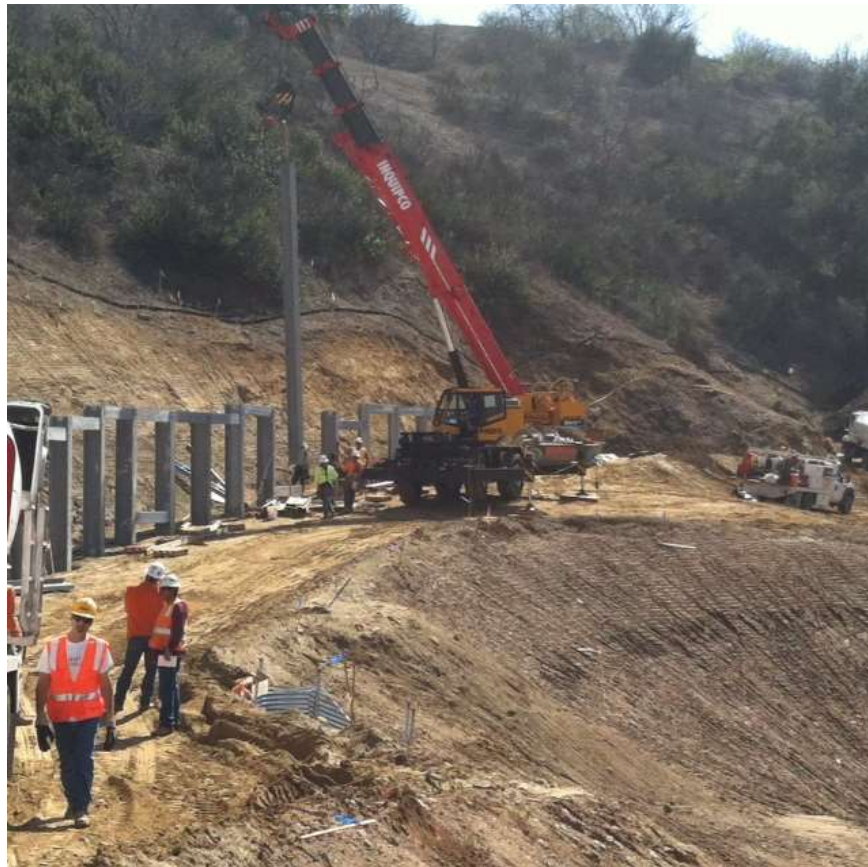
Figure 8: Union Construction crews continued road grading and retaining wall installation at Tower M57-T1 in Tonner Canyon, Segment 8, Phase 1.
