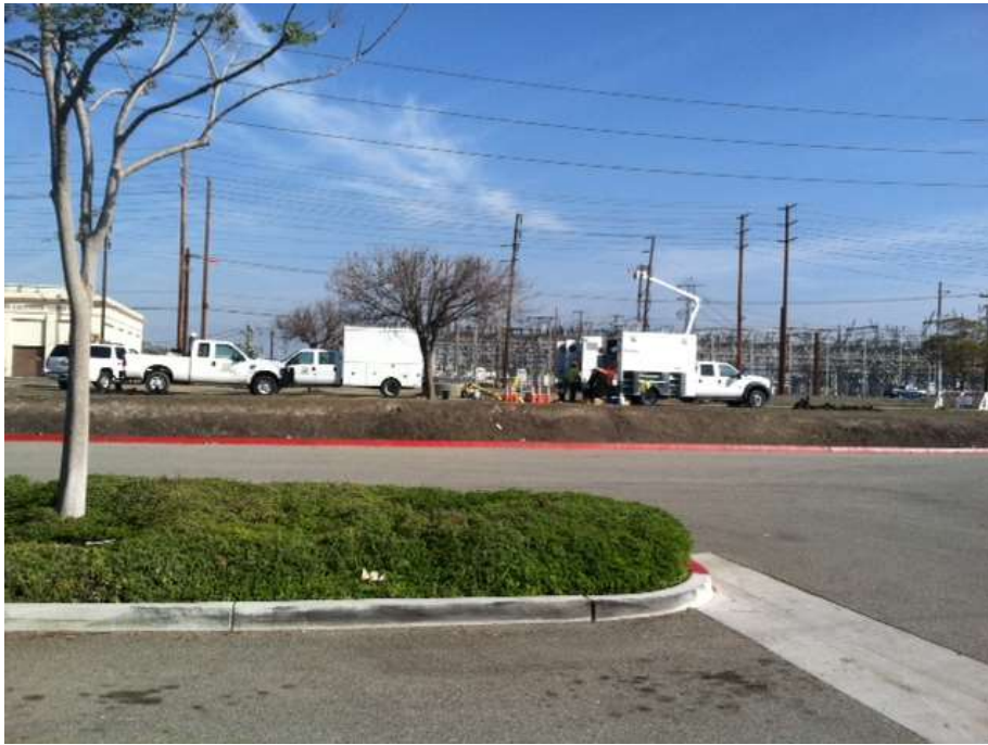
Figure 7: SCE crews pulling cable through underground vaults along Edison Avenue in the City of Chino.
