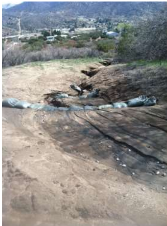
Figure 6: Runoff and sediment build up in drainage area adjacent to Juniper Ridge Road, as a result of Construct 5, Segment 6A slope.
