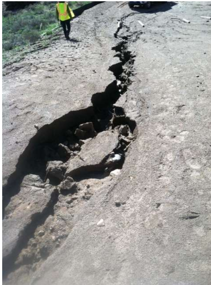
Figure 4: Gullying shown along the slope below Construct 5, Segment 6A.
