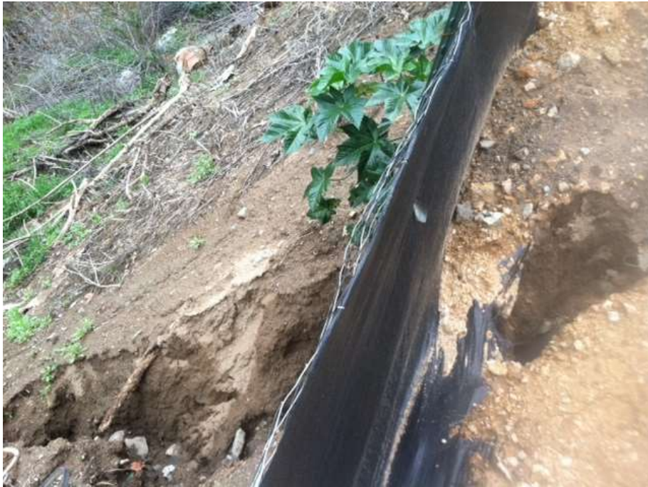
Figure 1: Erosion at soil storage area adjacent to the southern entrance to Loop Road L, Segment 6C.
