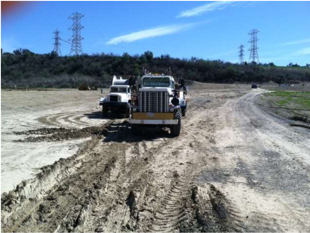
Figure 7: Construction vehicles were observed parked in an unapproved area on Segment 8, Phase 4.
