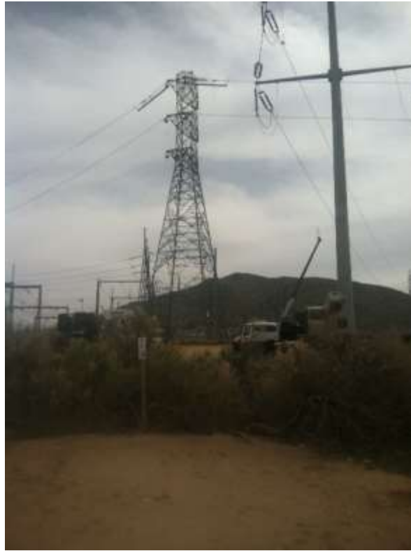
Figure 1: Tower assembly and wire work conducted on Segments 6 and 11 during an outage of adjacent lines.
