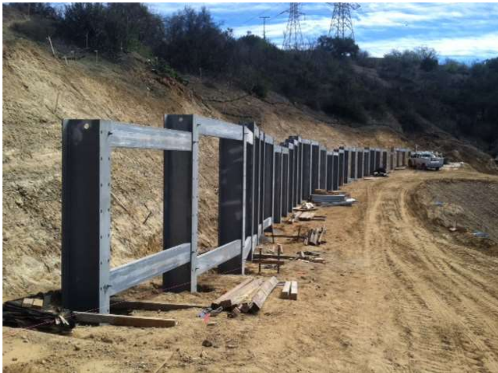
Figure 4: Wall construction along the access road for Tower M57-T1 in Tonner Canyon, Segment 8, Phase 1.
