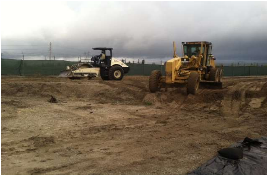
Figure 9: KGC developing a previously undisturbed portion of the Rancho Vista Materials Yard in preparation for material storage for the CHUG work.
