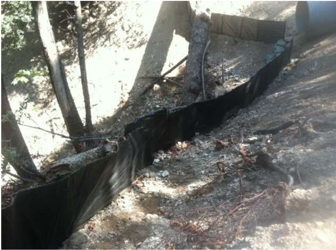
Figure 3: Silt fence and erosion repaired at Loop Road L at Mile 8.0.
