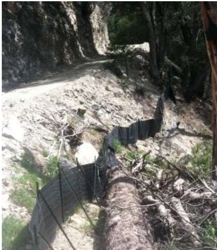
Figure 5: Silt fence repaired on Loop Road L at Mile 6.0. Housekeeping issues were identified to the PE present; damaged silt fence remained onsite and appears to be buried by new fencing install.
