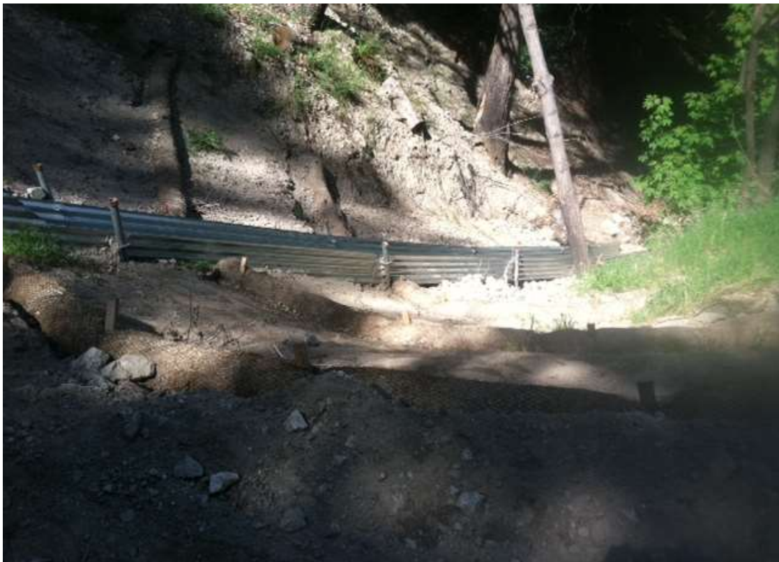
Figure 4: Straw wattles and slope have been repaired on Loop Road L Mac Drain at Mile 6.5.
