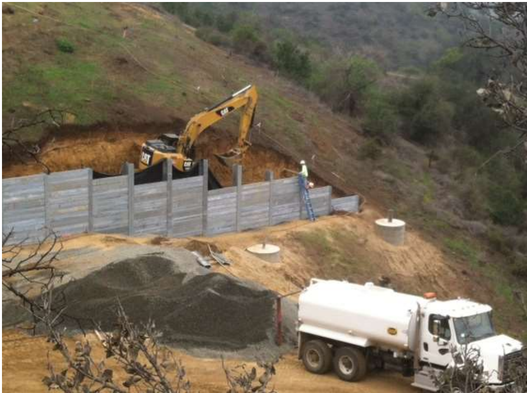
Figure 7: Union Construction crews continued road grading, placing drain material, and retaining wall installation, Tower M57-T1, Segment 8, Phase 1.
