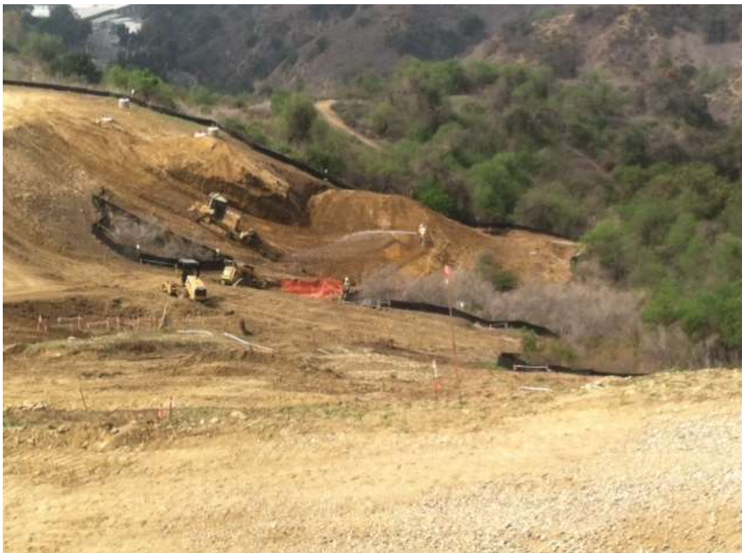
Figure 8: Patriot Construction crews continued excavation activities, including trenching, pipe and fill placement, and grading work at Tower M43-T3, Segment 8, Phase 4.
