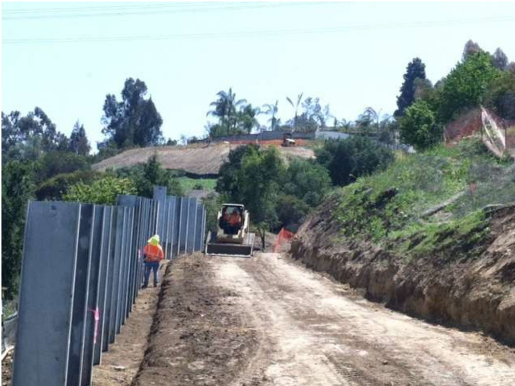
Figure 9: Patriot crews continued construction activities on the soldier pile wall for the access road to Tower M49-T, Segment 8, Phase 4.
