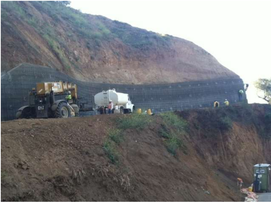
Figure 7: Union crews continued work on the soil nail wall at Tower M27-T3 in Duarte, Segment 7.
