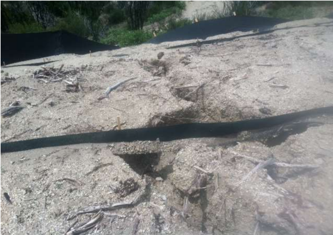
Figure 3: Gullying damage seen at Pull/Tensioner Site 62/63, Segment 6.
