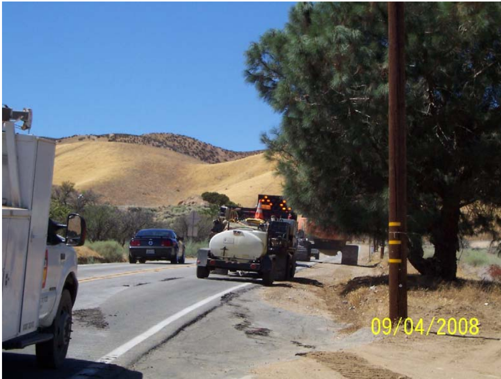
Figure 3: Damage to asphalt during transport of the auger machine along 110 th Street.
