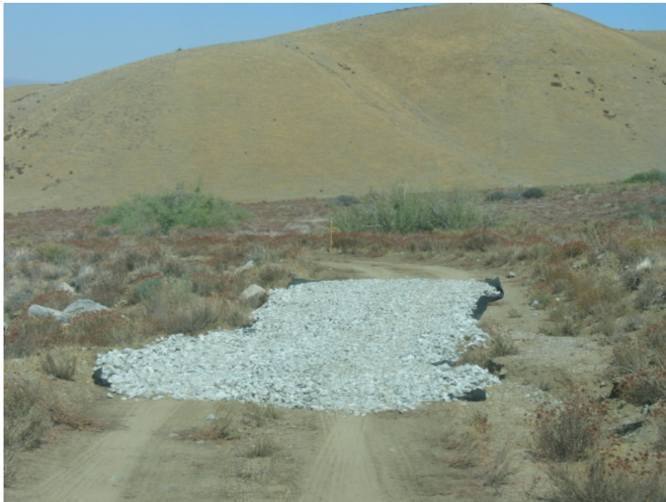
Figure 4: Installation of fabric and rock to protect a drainage crossing an access road in Section 3.
