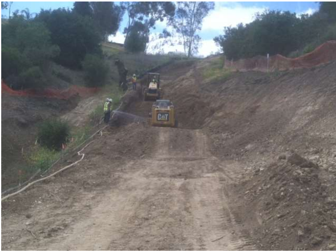
Figure 5: Construction activities continued on the soldier pile wall for the access road to Tower M49-T1, Segment 8, Phase 4.
