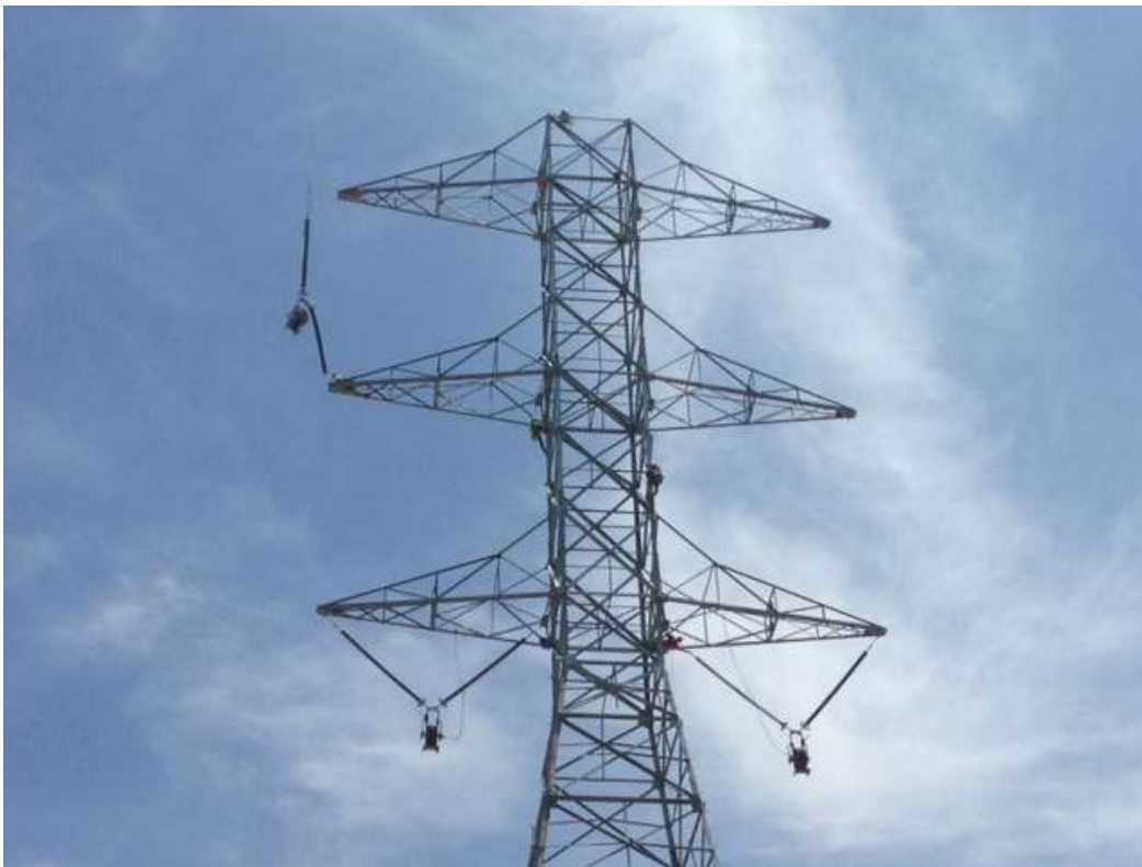
Figure 6: Material delivery via helicopter to towers along Segment 7 in preparation for conduction installation.
