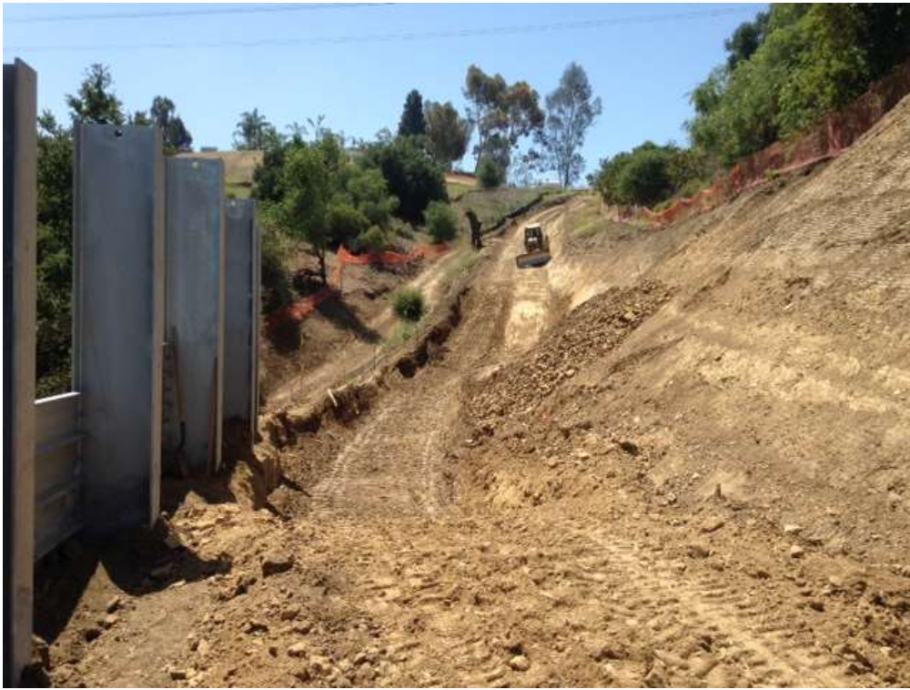
Figure 9: Patriot crews continue grading the access road and Hilfaker wall construction at Tower M49-T1, Segment 8, Phase 4.
