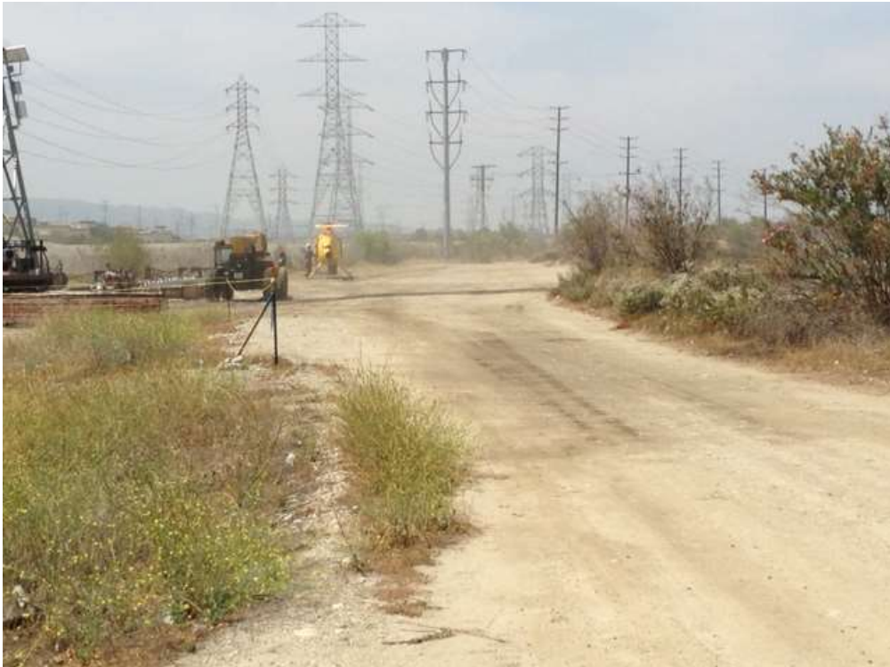
Figure 10: CPUC EM observed a PAR helicopter conducting operations from an access road outside of approved disturbance limits, Segment 8, Phase 4. During these operations large amounts of fugitive dust was observed leaving the area as it was not watered prior to the work beginning.
