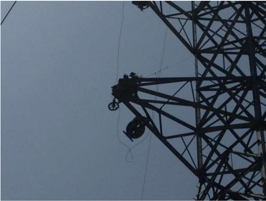
Figure 11: Inactive, vacant raptor nest removal from an arm of Tower M43-T1, Segment 8, Phase 4. The CPUC EM was onsite for the removal and observed the proper protocol was observed for the duration of the removal.
