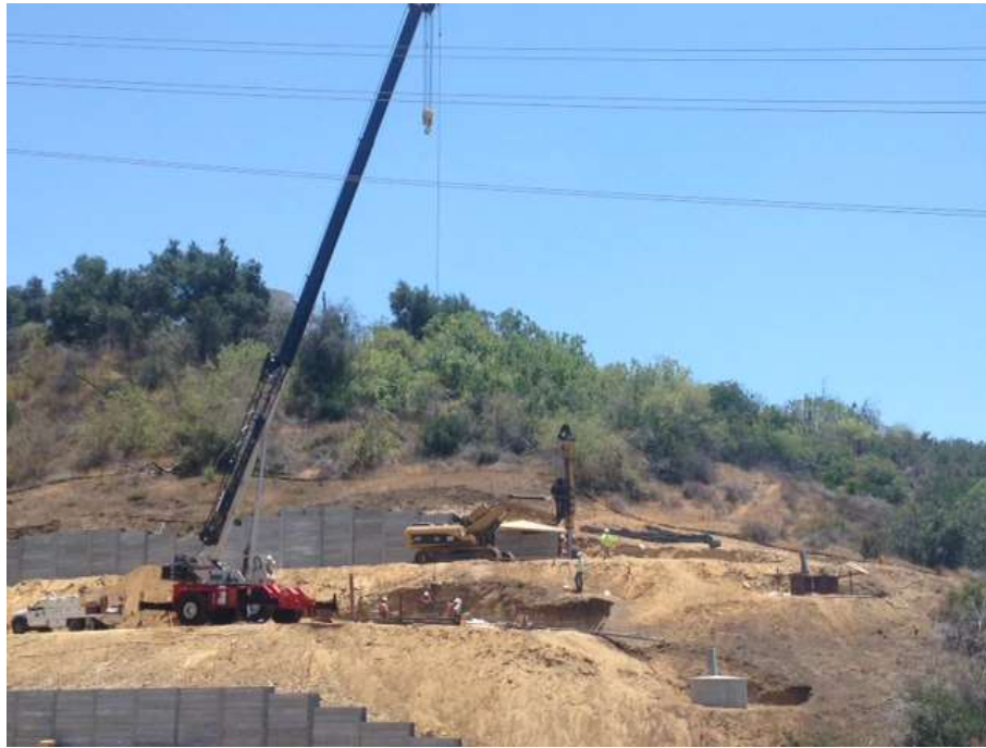
Figure 7: Foundation drilling and wall construction at Tower M57-T1 in Tonner Canyon, Segment 8, Phase 1.
