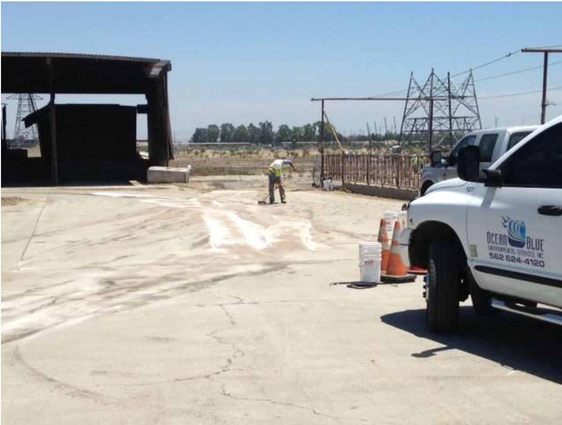
Figure 9: Clean-up of hydraulic spill caused by a broken hose on a street sweeper, Segment 8, Phase 3.
