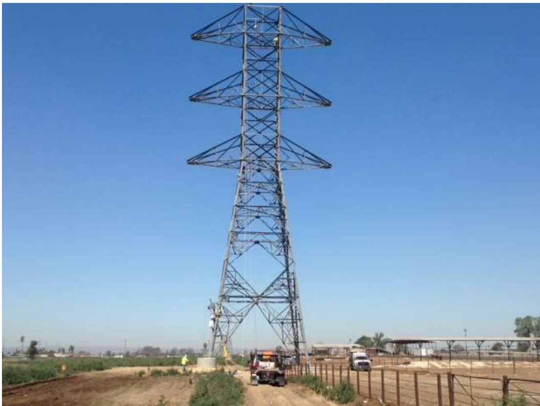
Figure 6: Tower erection and installation of FAA lighting at Tower M70-T3, Segment 8, Phase 3.
