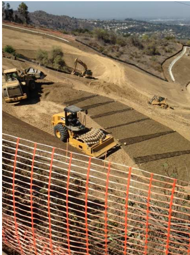
Figure 8: Crews working on the installation of geogrid for landslide repairs at Tower M43-T3, Segment 8, Phase 4.
