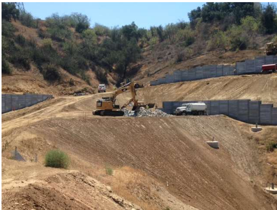
Figure 4: Grading and wall construction at Tower M57-T1 in Tonner Canyon, Segment 8, Phase 1.
