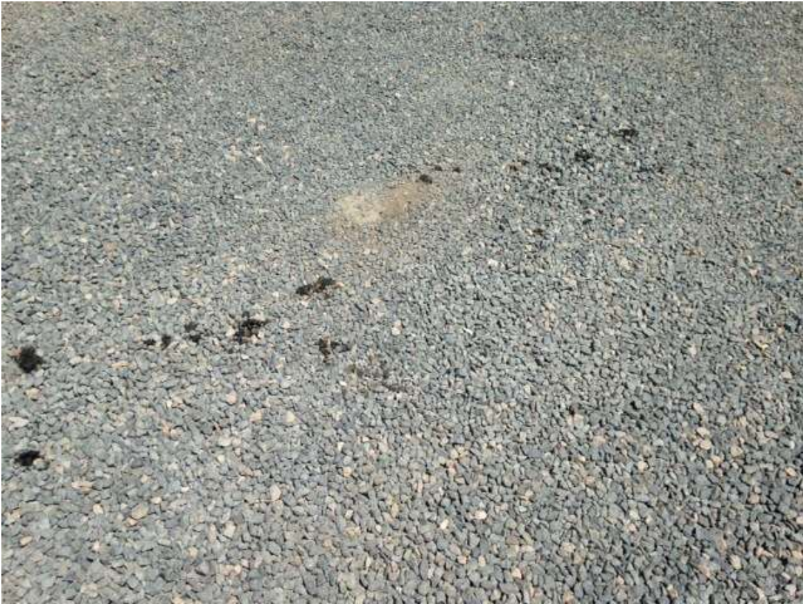
Figure 13: The CPUC identified a hydraulic leak from construction equipment near Tower M66-T1, Segment 8, Phase 3.
