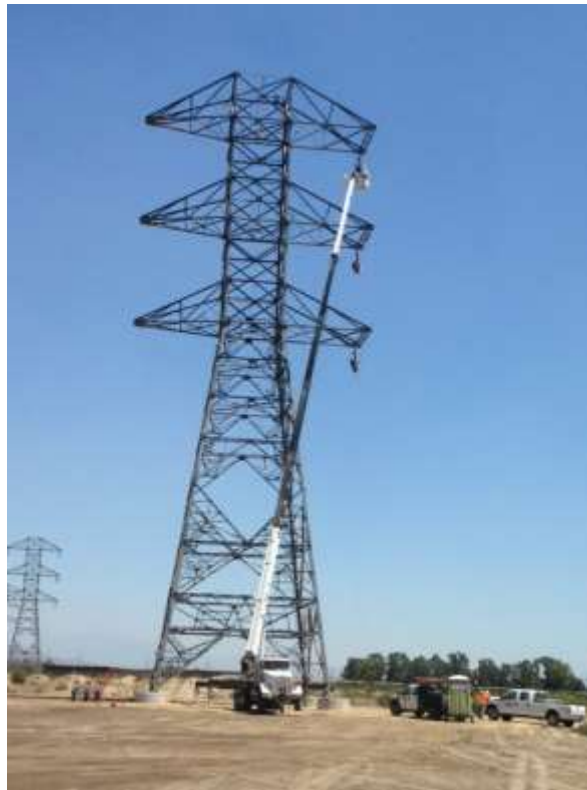
Figure 7: Henkels and McCoy crews installed Travelers and blocks at Towers M68-T5 through M73-T4, Segment 8 Phase 3.
