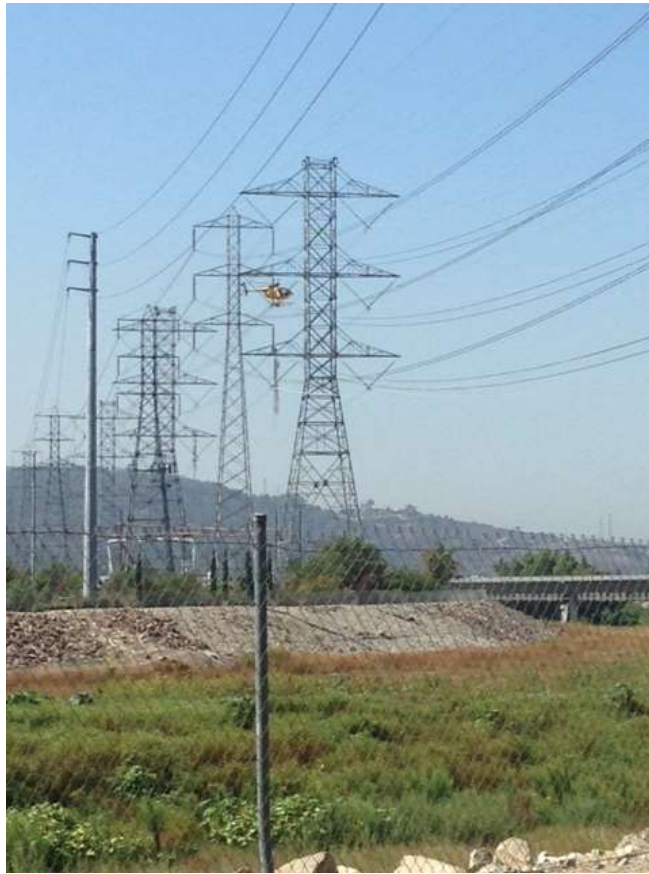
Figure 5: Wire repair work conducted at Towers M27-T2 through M27-T4 and M28-T3, Segment 7.
