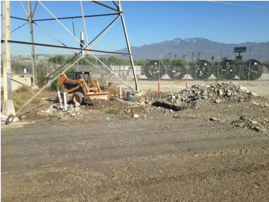
Figure 4: PAR conducted conduit/vault installation from Tower M31-T4 through M59-T1D to the Rio Hondo Substation, Segment 7.
