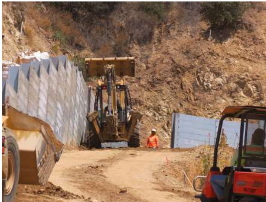
Figure 8: An SCE biologist observed two loaders from Union Engineering transporting soil and placing it in the roadbed where Jurisdictional waterway crosses the road, without a full-time monitor present. This incident was observed at Tower M27-T3 on Segment 7. Photo courtesy of FRED.
