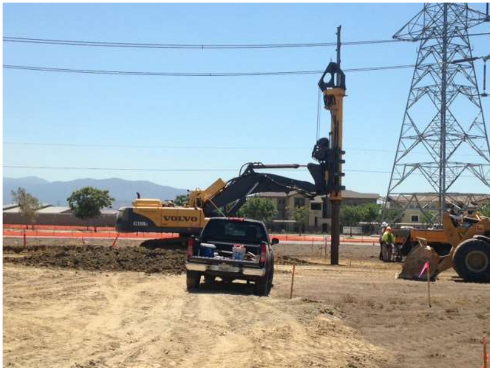
Figure 6: Henkels and McCoy crews continued foundation installation activities at Towers M6-T3A, Segment 8 Phase 3.
