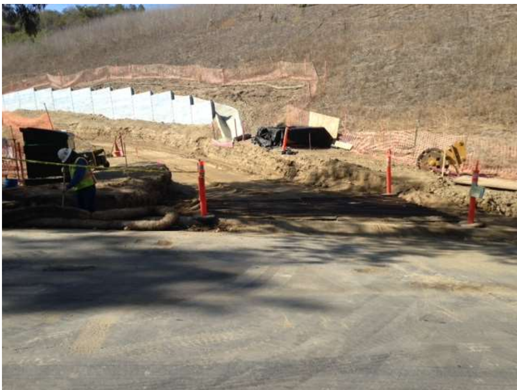
Figure 6: V-ditch and BMP installation work along the access road to Tower M49-T1 in Segment 8, Phase 4.
