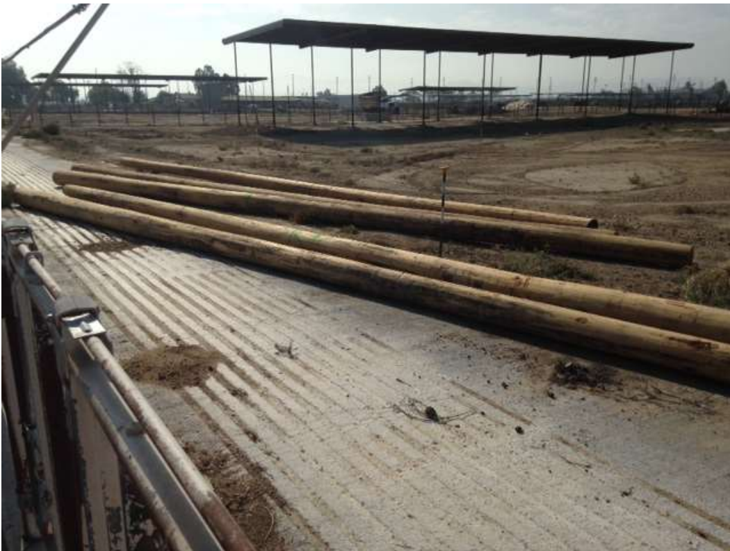
Figure 8: TRTP materials (guard poles) staged outside of approved work limits, Segment 8, Phase 3.
