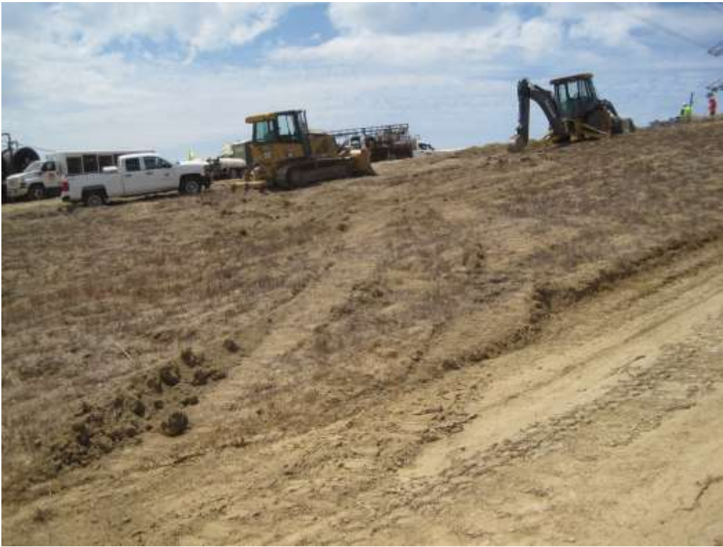
Figure 7: Tracks from a project grader observed outside of approved work limits, Segment 8, Phase 4. (Photo courtesy of FRED)
