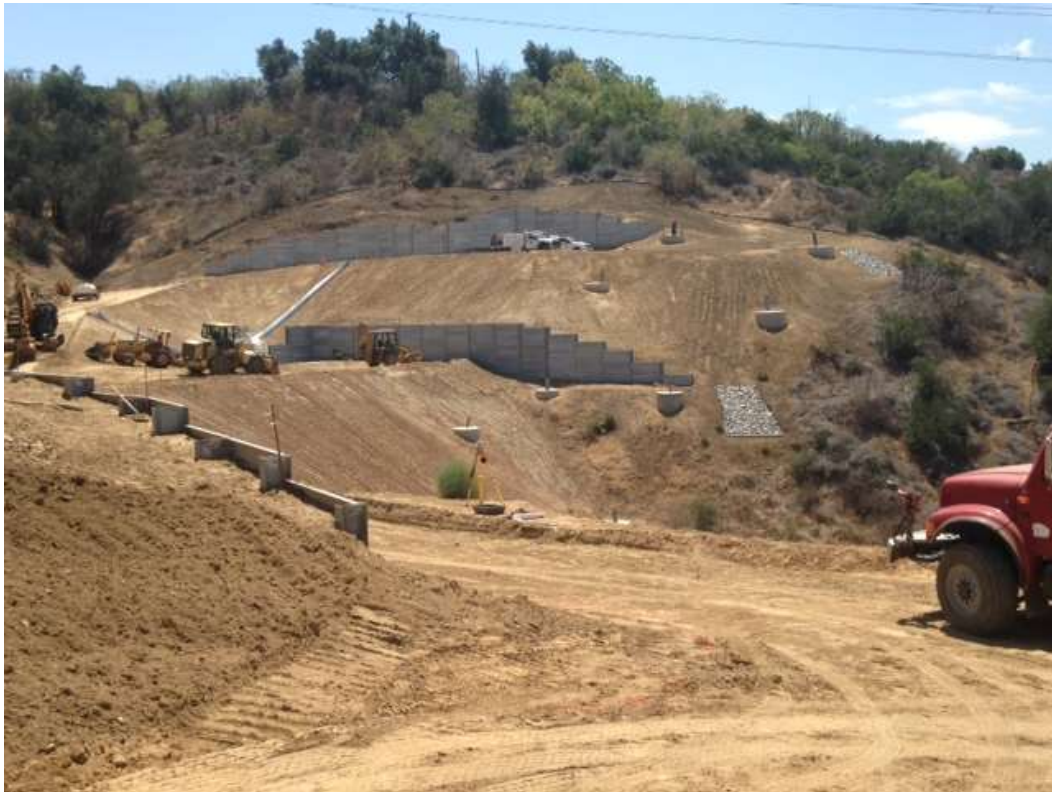
Figure 5: Soil import and benching work along access road to Tower M57-T1, Segment 8, Phase 1.
