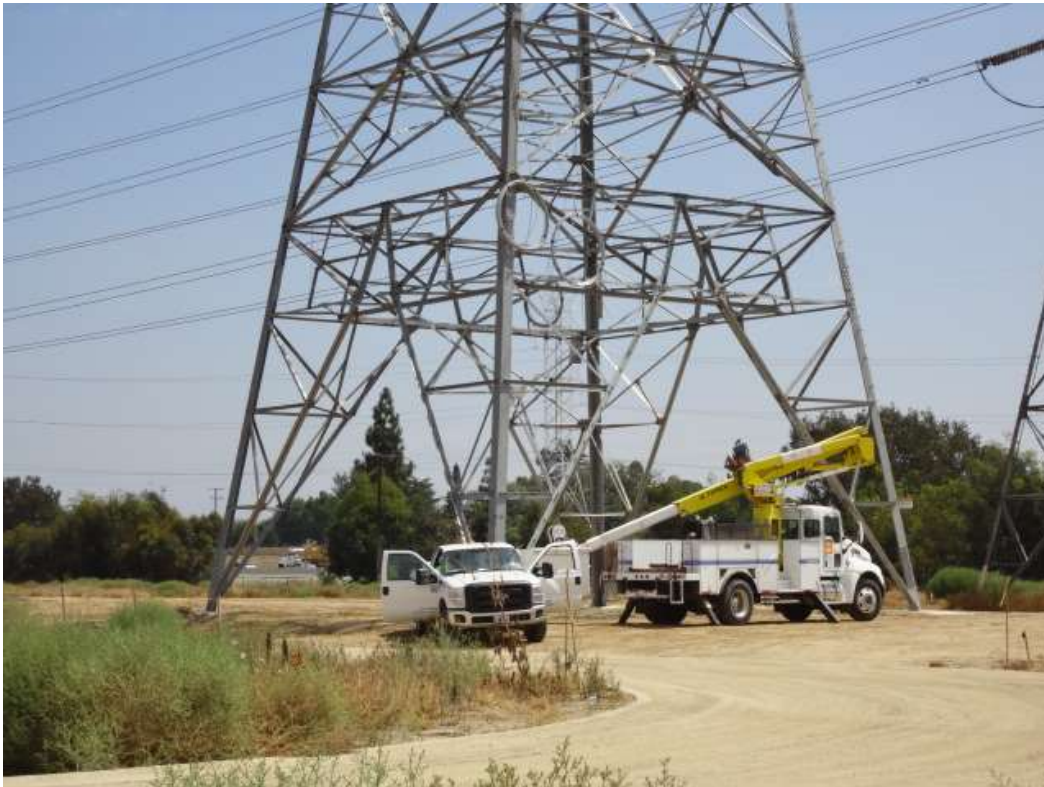
Figure 4: Wire splicing work near the Rio Hondo Substation, Segment 7. (Photo courtesy of FRED)
