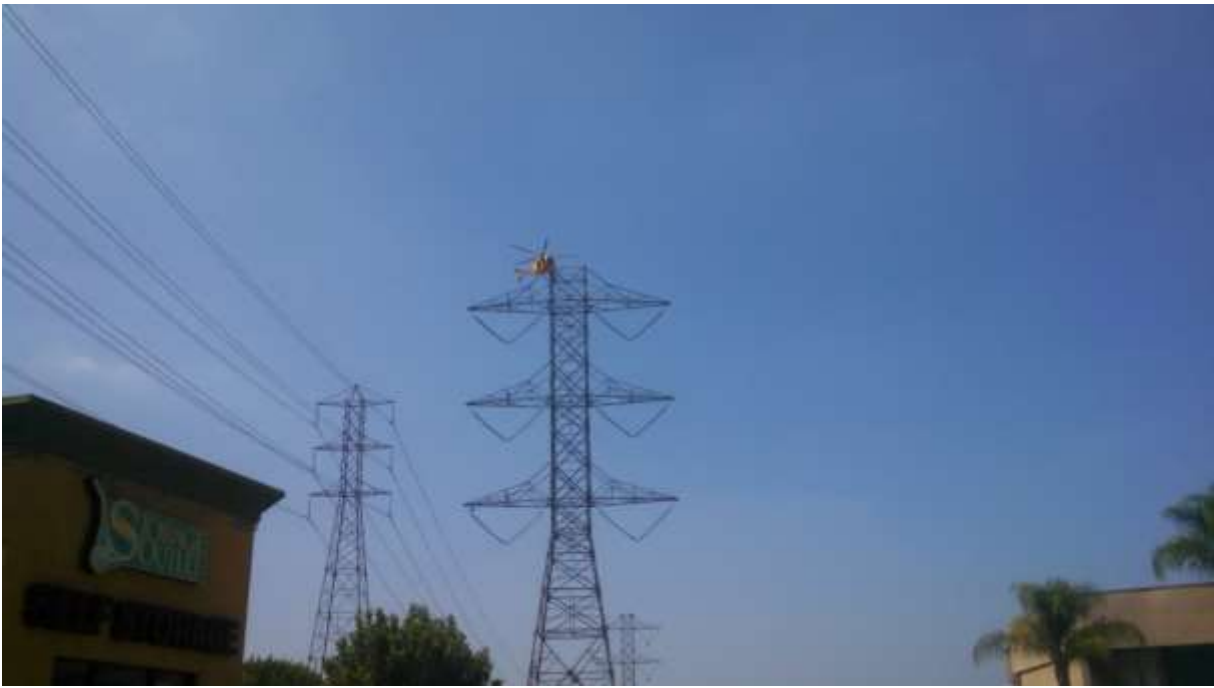
Figure 3: A worker was observed dropping a tool while stepping onto a tower from the helicopter at Tower M38-T2, Segment 7.
