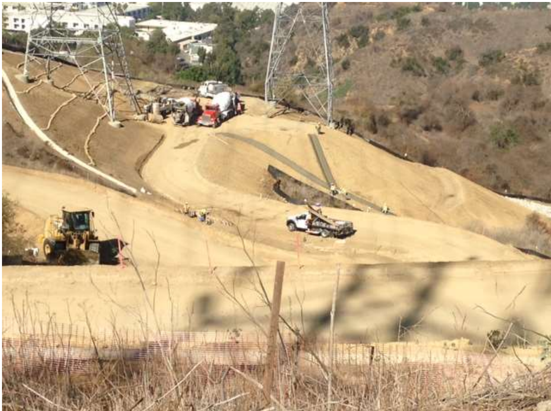
Figure 6: Patriot completed final grading and v-ditch installation at Tower M43-T3, Segment 8, Phase 4.
