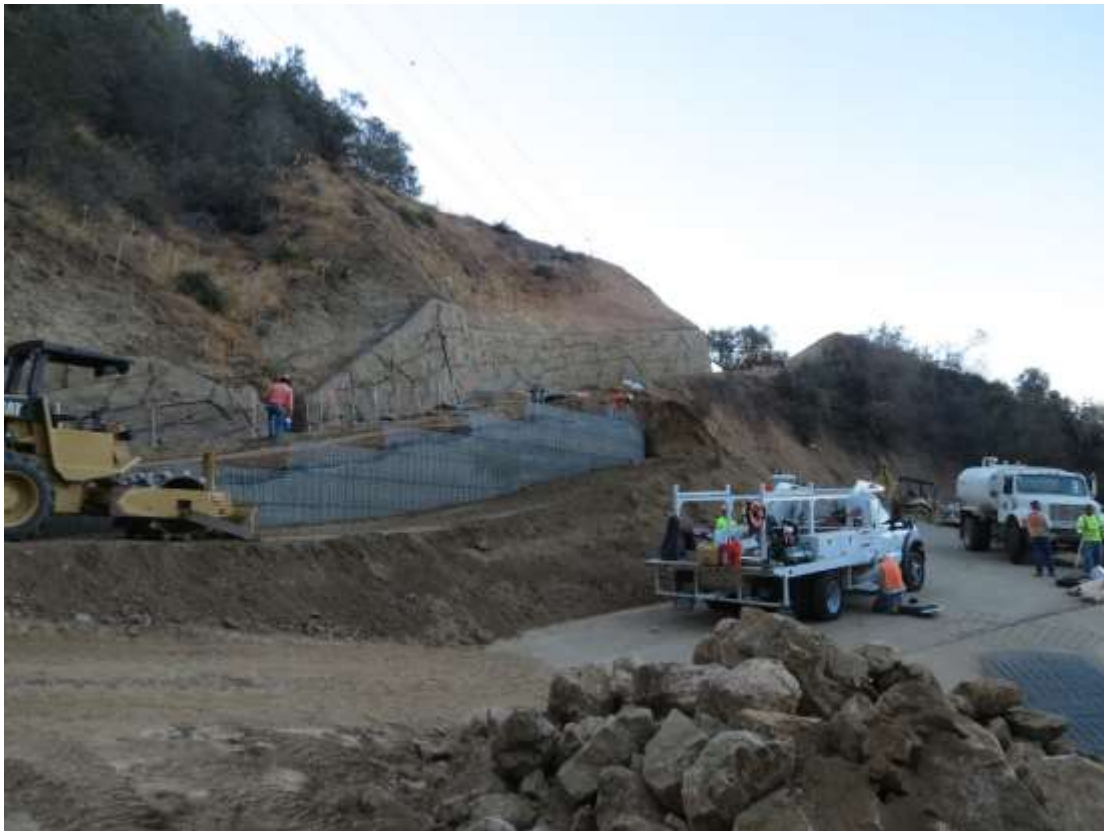
Figure 4: Union Engineering continued work on the support wall along the access road to Tower M27-T3 in Duarte, Segment 7.
