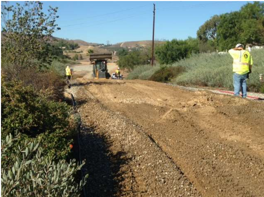
Figure 8: Power Grade installed rock for roadway entrances to the CHUG right-of-way in Chino Hills.
