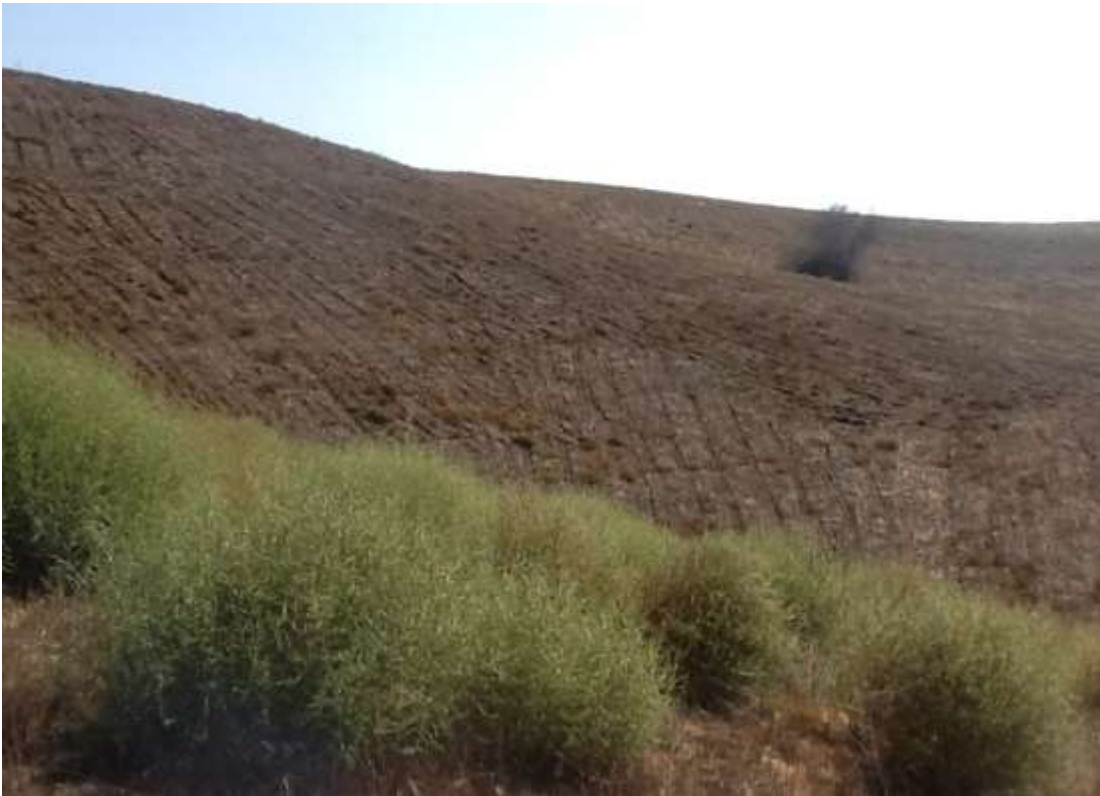
Figure 3: Vegetation removal at the future site of the Western Transition Station, Chino Hills Underground.
