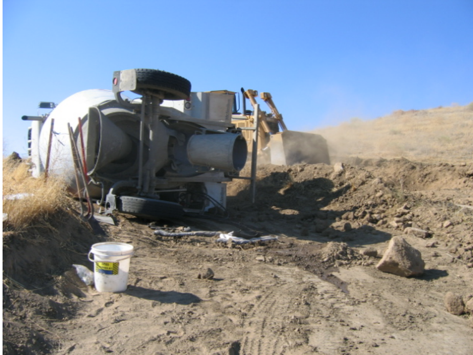
Figure 1: Overturned cement truck in Section 3, September 10, 2008.
