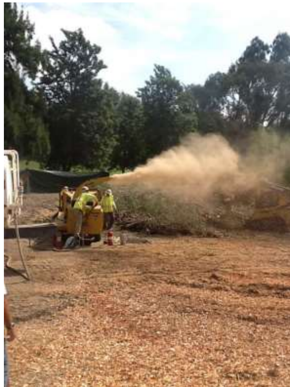
Figure 6: Vegetation removal along the CHUG right-of-way at VC #2. Vegetation was chipped and distributed on site.
