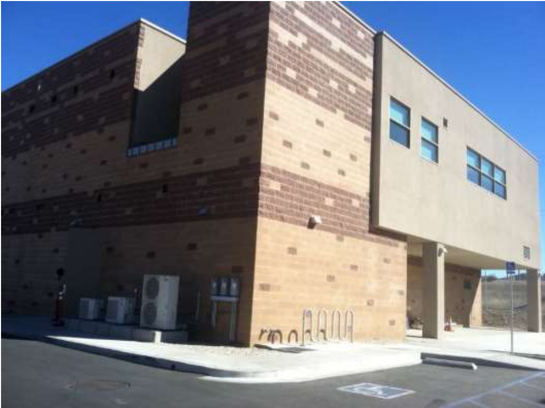
Figure 1: Construction of the control building at the Vincent Substation is nearing completion.
