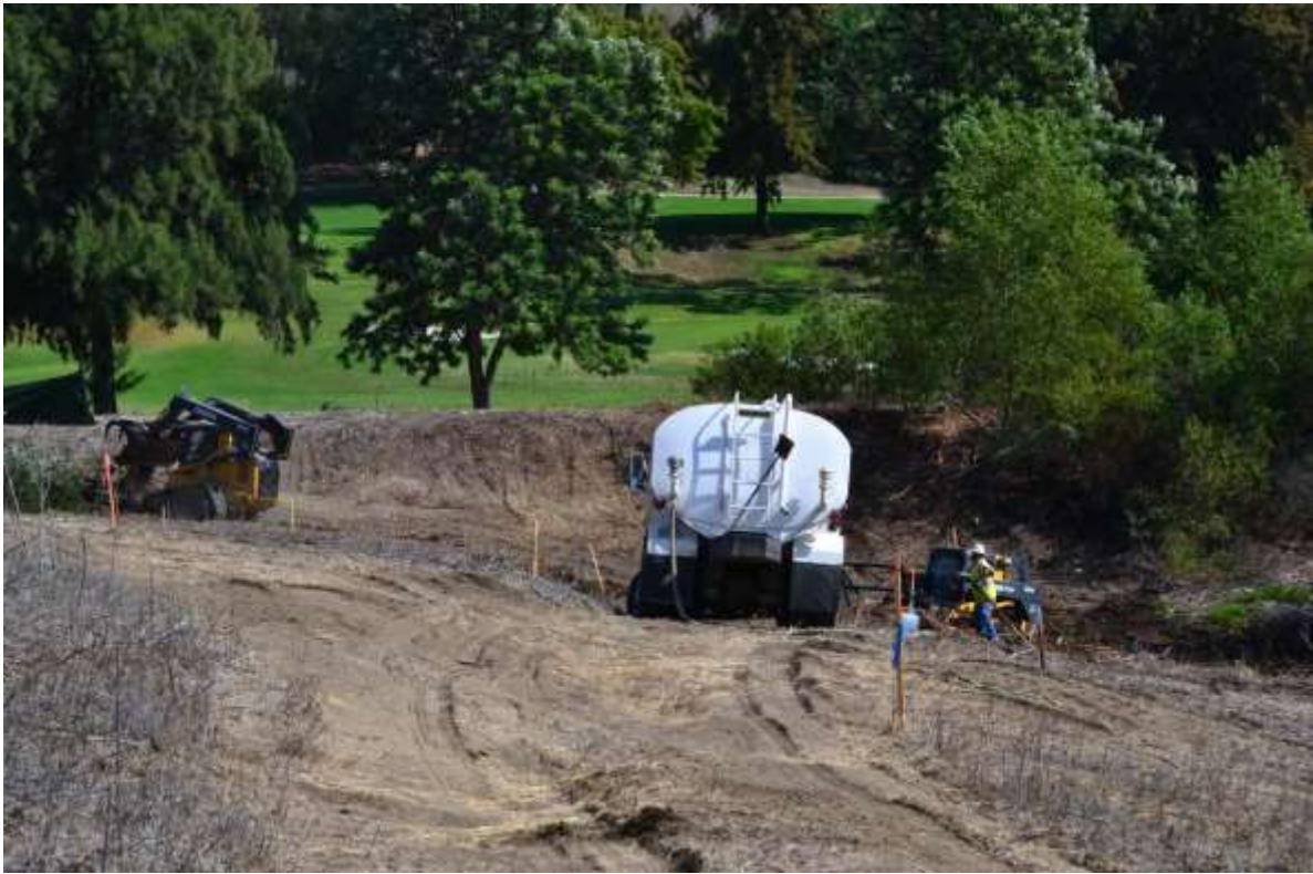
Figure 9: Clear and grub crews continue to clear vegetation at VC #2 along the CHUG right-of-way.
