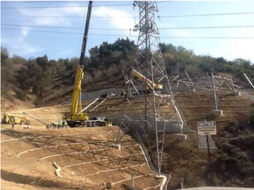
Figure 7: Assembly and erection of Tower M24-T1A adjacent to M57-T1 in Tonner Canyon, Segment 8, Phase 1.
