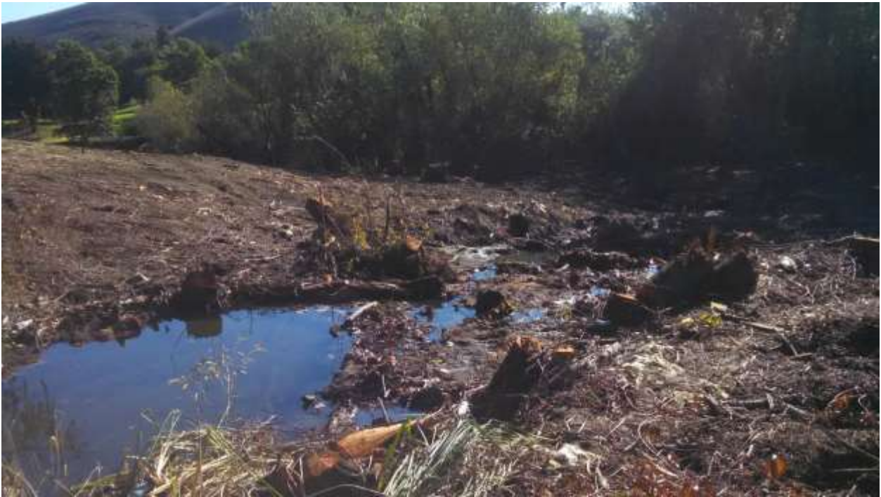
Figure 5: Standing water is present near VC #2 in Chino Hills. The contractor is reviewing plans for diverting the water during construction of the underground infrastructure.
