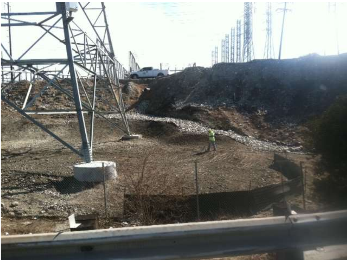
Figure 4: Tower areas being recontoured along the 605 Freeway near the Rio Hondo Substation, Segment 7.
