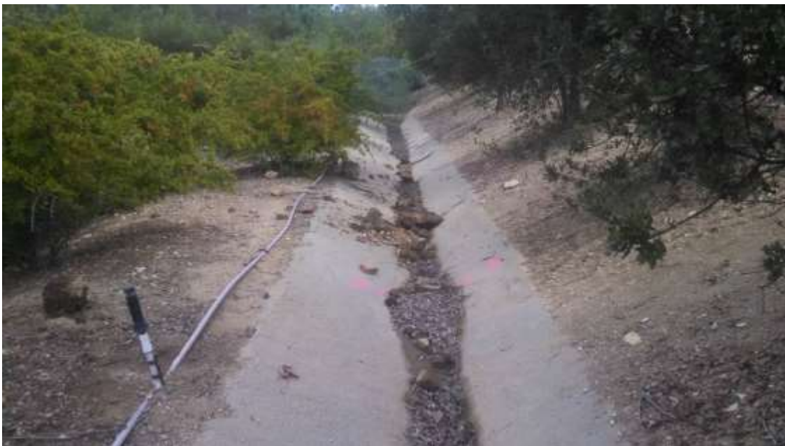
Figure 2: Erosion of loose soils from the CHUG WTS was observed outside of approved disturbance areas and into concrete v-ditches.
