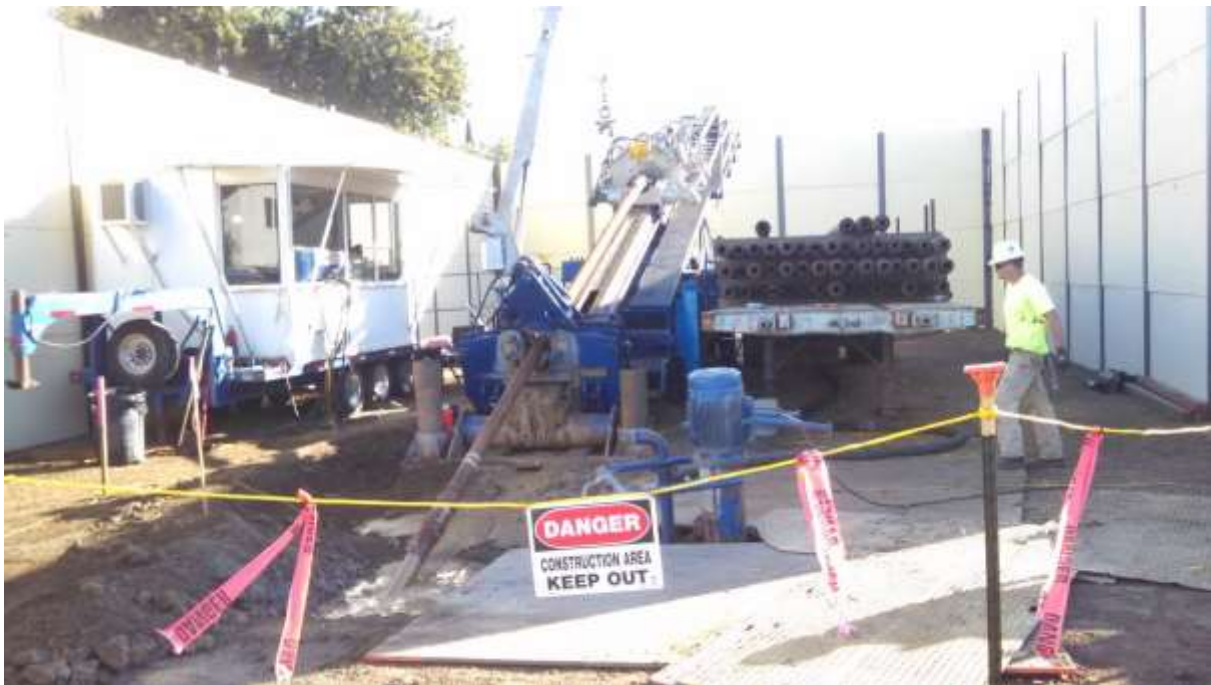
Figure 2: HDD pilot drilling at the first bore location in the City of Chino.
