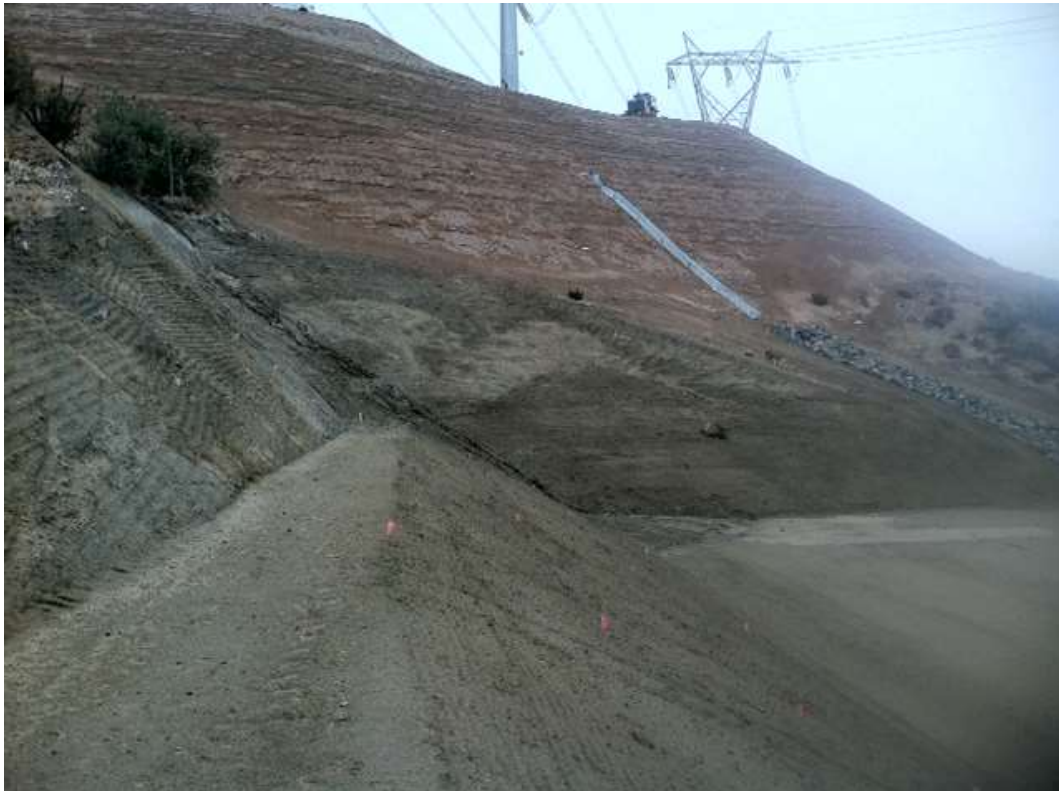
Figure 2: Slope of Construct 5, Segment 6A, post-storm.
