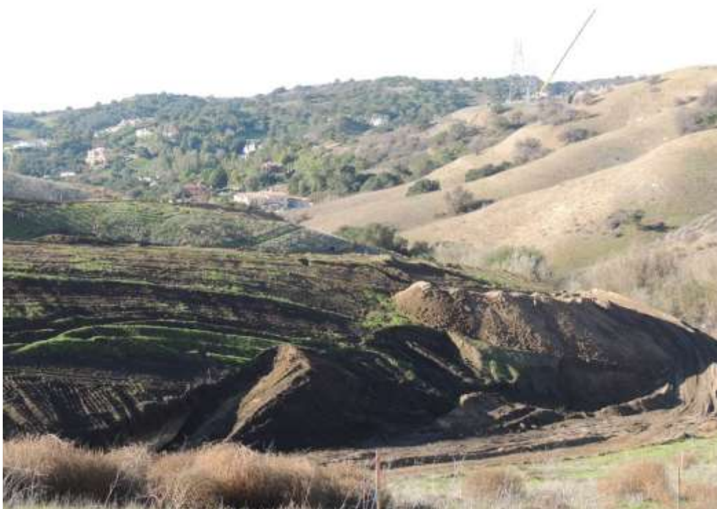
Figure 4: Grading is in process at the Western Transition Station at the west end of the Chino Hills Underground alignment.
