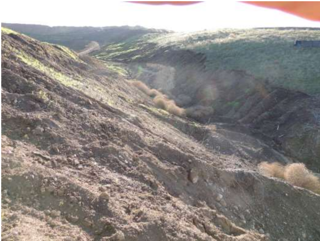
Figure 5: Storm damage and erosion after recent rains at the Western Transition Station.
