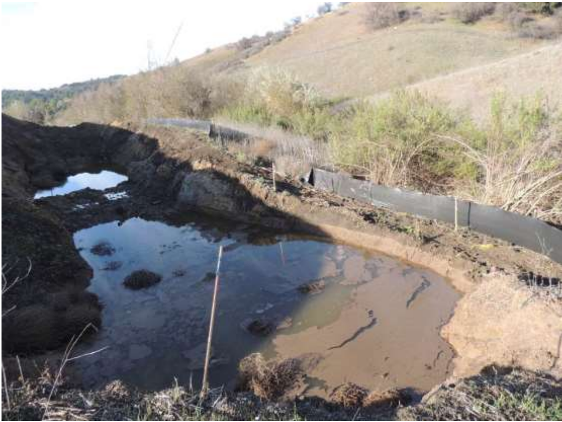
Figure 5: Keyway excavations at the work boundary of the WTS. The keyway excavations acted as sediment traps during the recent storms.
