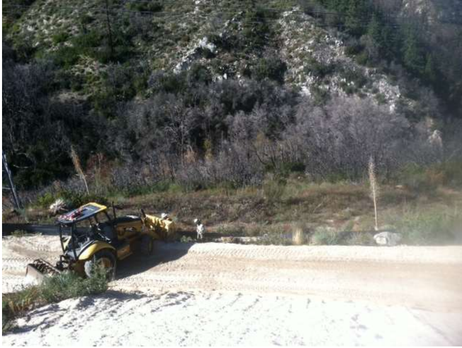
Figure 1: Post storm road cleanup and BMP perimeter maintenance at Construct 68, Segment 11C.
