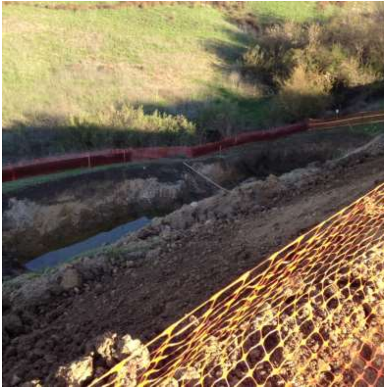
Figure 1: Before the holiday, the steep keyway excavations at the WTS were fenced and wildlife ramps were installed, Segment 8, 500 kV Underground (photo courtesy of SCE).
