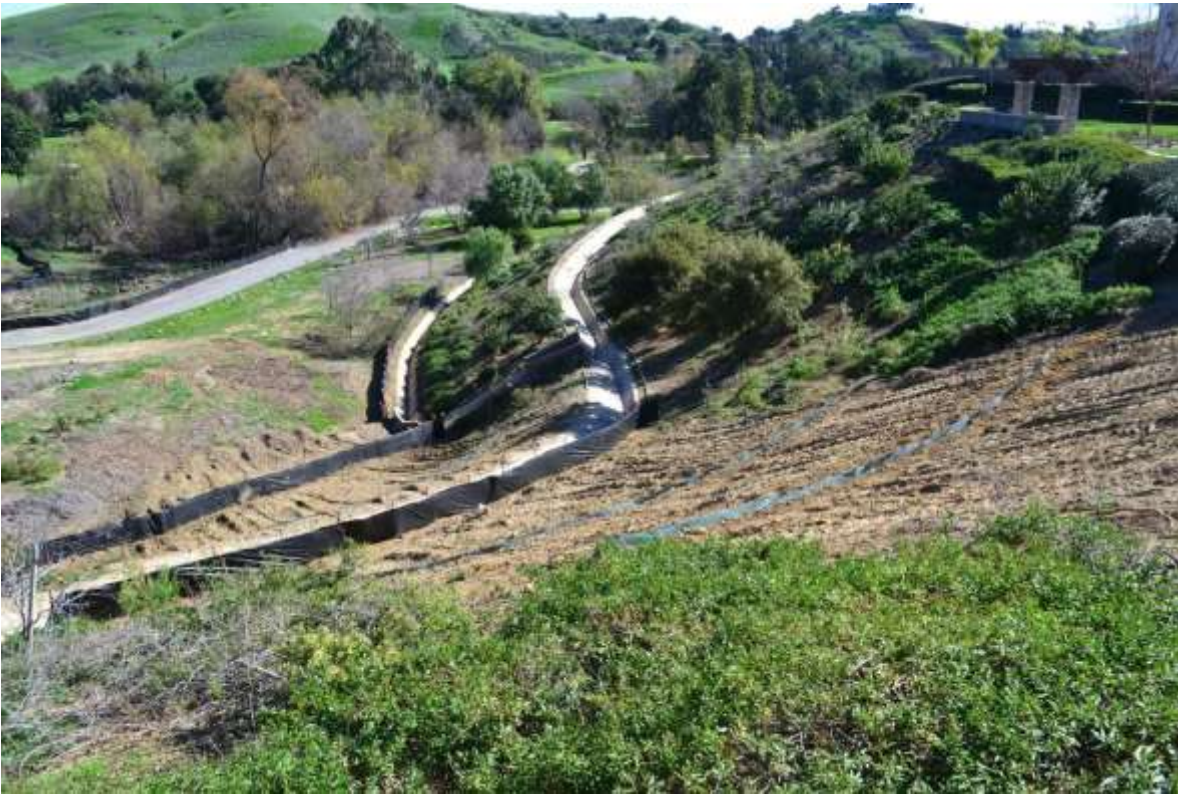
Figure 6: Additional BMPs have been installed on project disturbed slopes near VC #2, 500 kV Underground.
