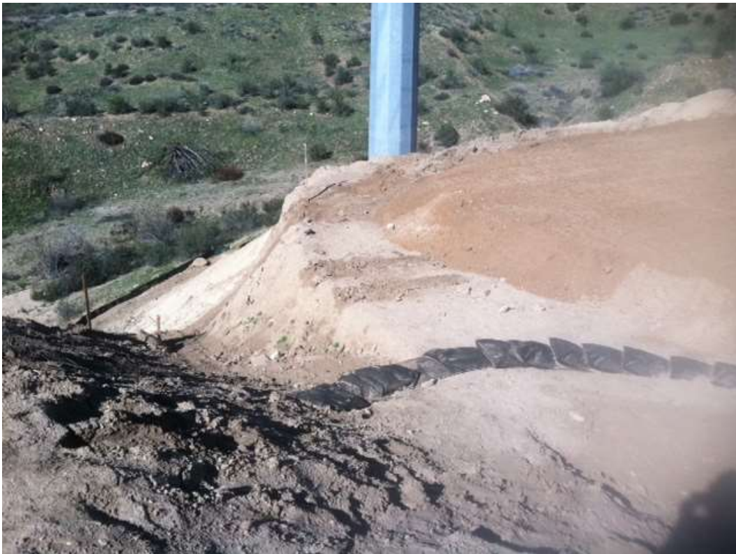
Figure 3: BMP installation that occurred at Construct 11AXXX on Segment 11C; additional BMPs were to be added to increase Jurisdictional Drainage protection at the toe of the slope.
