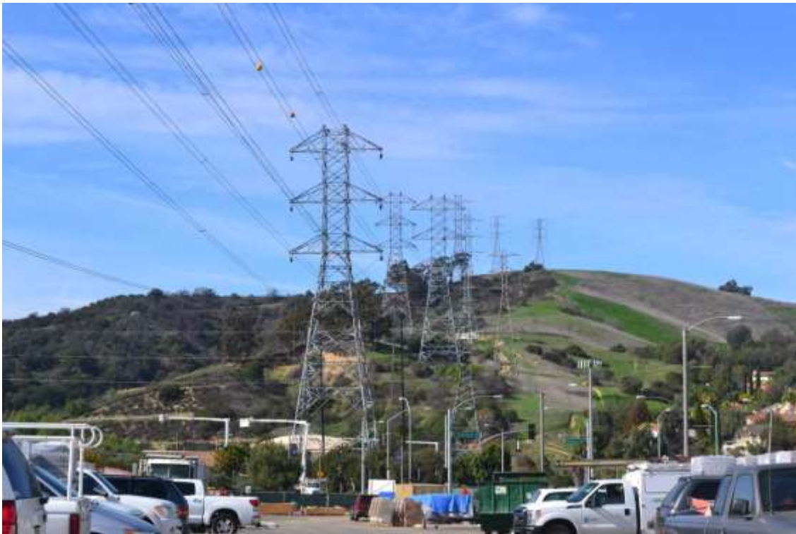
Figure 4: Wire installation between Towers M55-T2 and M47-T1 near Pathfinder Park, Segment 8, Phase 4.
