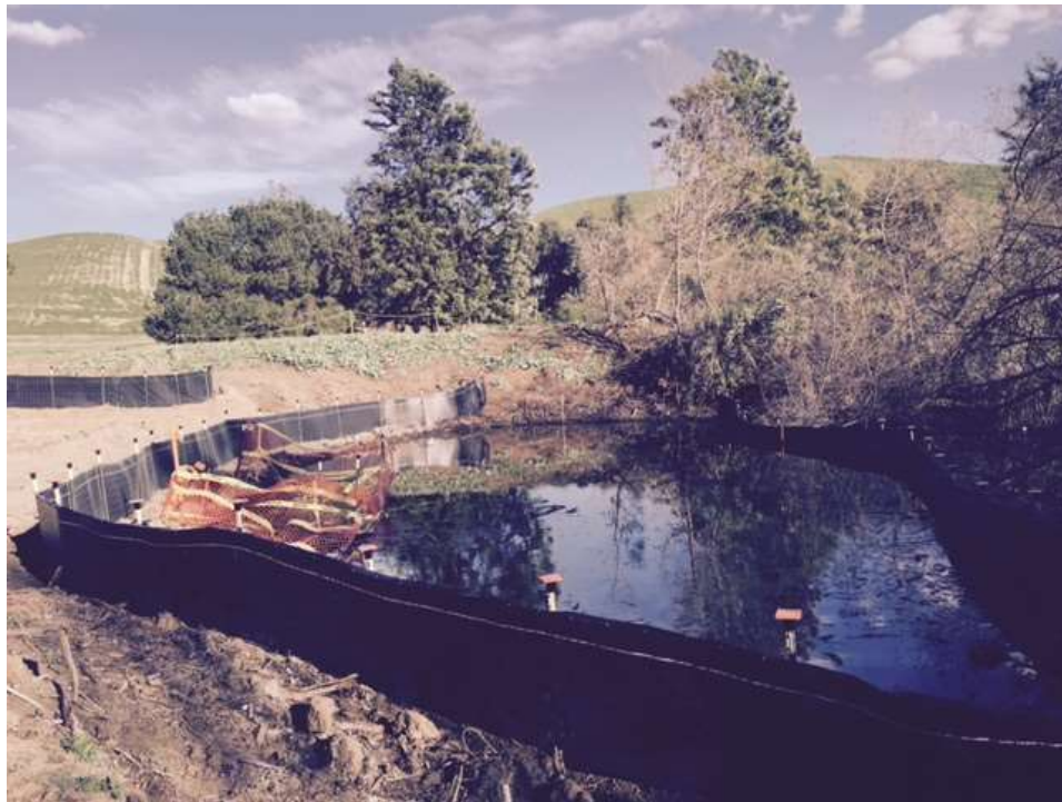
Figure 6: Silt fencing was installed at the edge of the 500 kV Underground right-of-way near VC #2 (pictured on right side) when no water was present. SCE will eventually install a gravel bag barrier to prevent water from entering the work area from the adjacent wetland.
