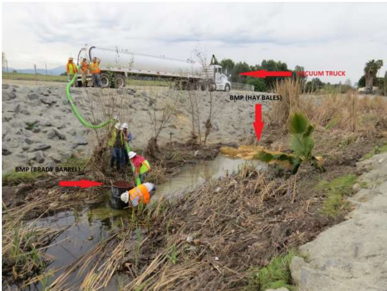
Figure 7: Cleanup of the frac-out in the Carbon Canyon Creek. The Brady barrel was installed to contain further drilling mud released into the creek. Hay bales were deployed downstream to contain drilling muds to the immediate area. The vacuum truck was used to remove the drilling muds that had settled on the creek bottom. Photo courtesy of SCE FRED.
