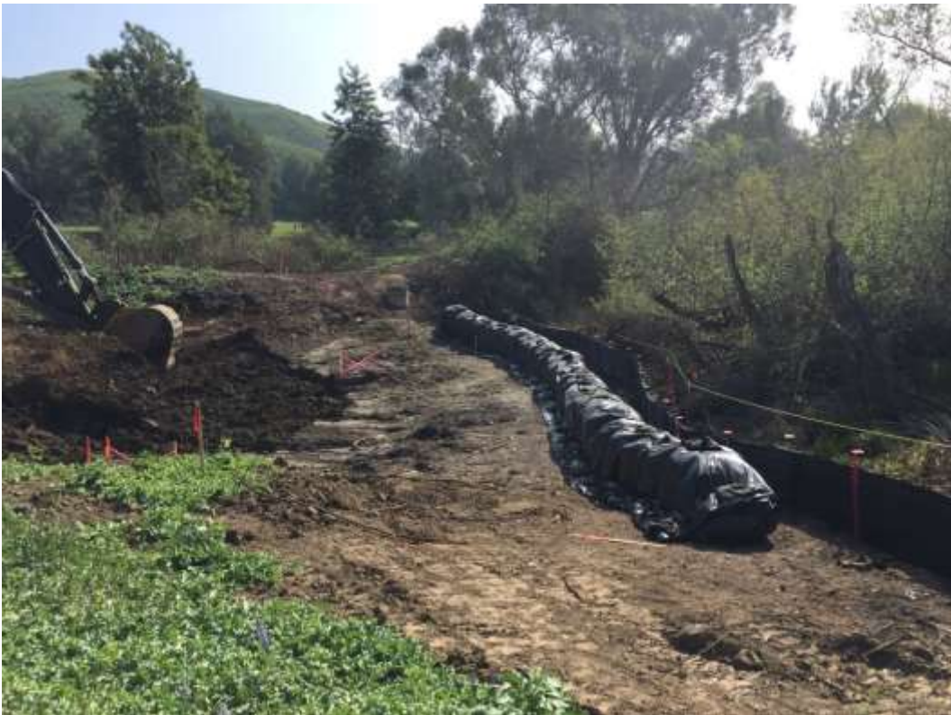
Figure 8: Installation of an impermeable barrier per Dewatering Plan of VC#2, 500 kV Underground.
