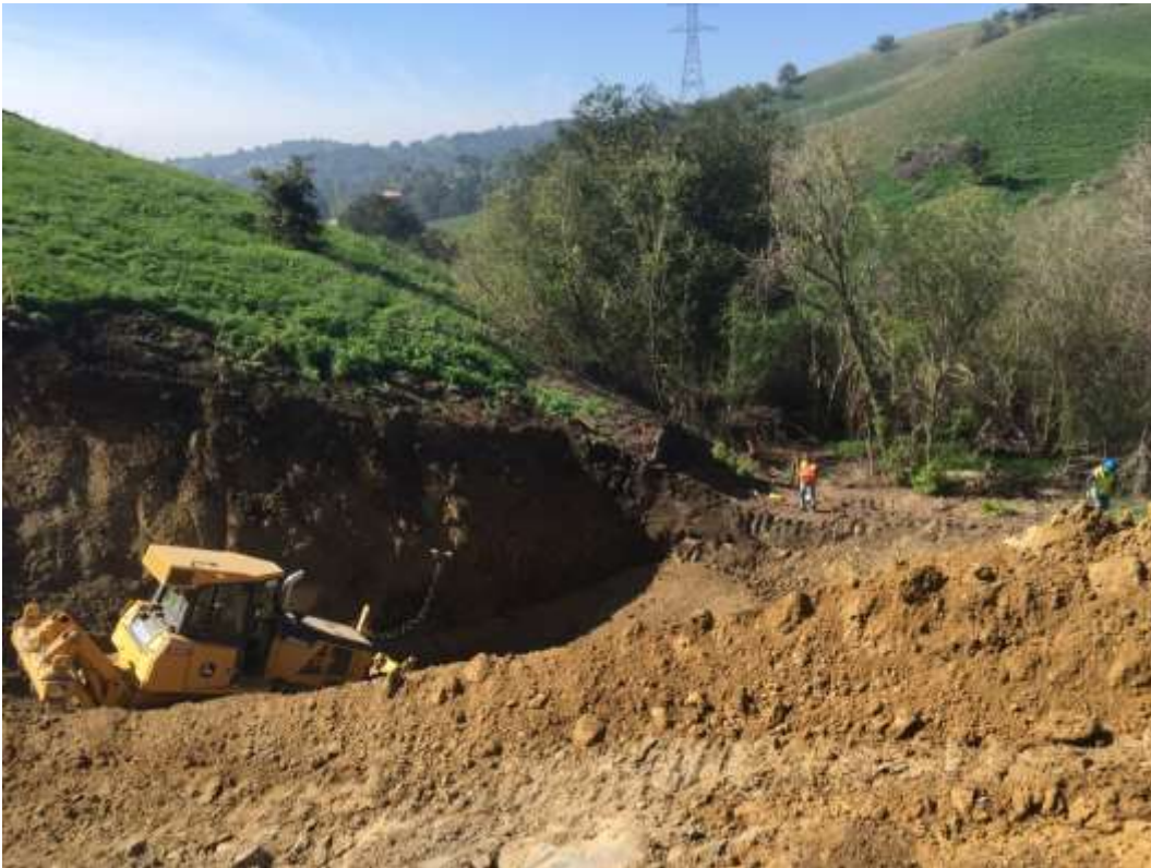
Figure 5: Grading and key excavations occurred in the middle canyon of the WTS, 500 kV Underground.
