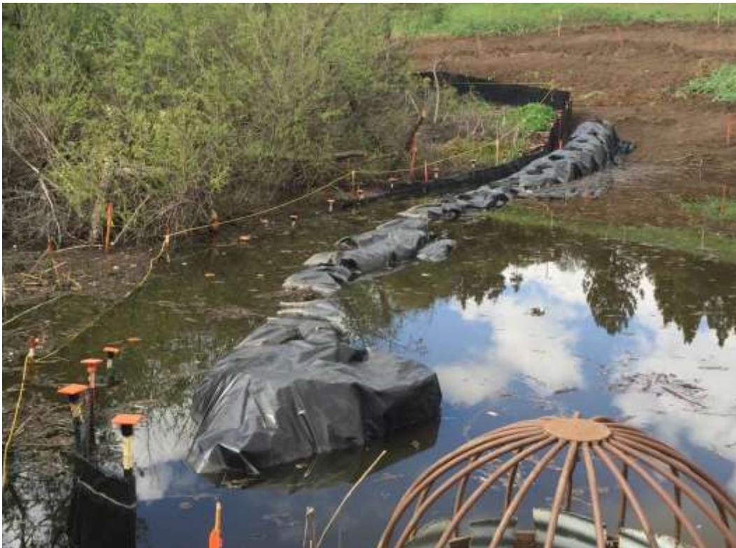
Figure 8: Water breaching the impermeable barrier and silt fence at VC #2, 500 kV Underground.
