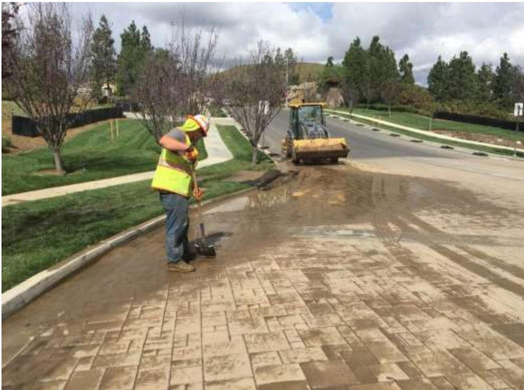
Figure 3: Crews working on post-storm clean-up along Canon Lane in Chino Hills, 500 kV Underground.
