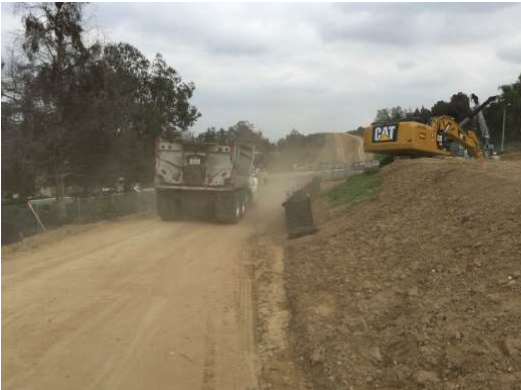
Figure 11: Excessive dust coming from access road to VC #6, 500 kV Underground.
