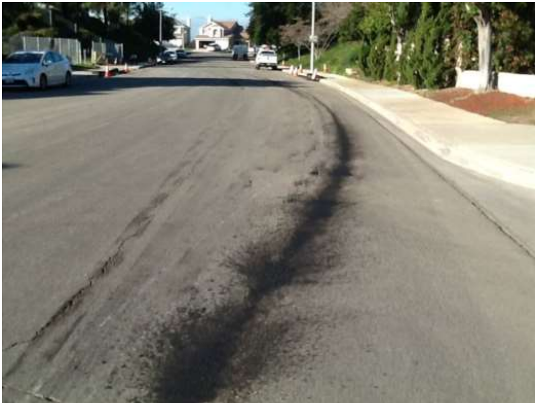
Figure 9: Oil spill along Lost Trails Drive, 500 kV Underground (photo courtesy of SCE).
