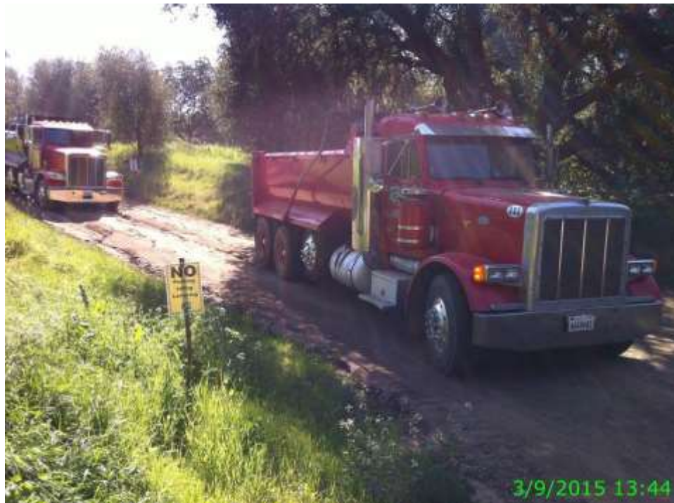
Figure 4: Dump trucks idling within exclusion zone for nesting birds on Segment 8, Phase 4 access road. Note signs prohibiting idling in the nesting bird buffer (photo courtesy of SCE).
