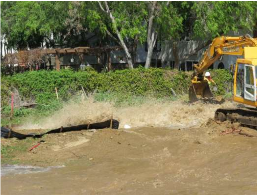
Figure 5: Rupture of the 15-inch City of Chino Hills water line during HDD operations (photo courtesy of SCE).
