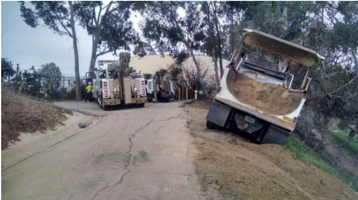
Figure 9: Dump truck off of approved road limits and load spilling between Towers M49-T4 and M50-T1 (Segment 8, Phase 4) (photo courtesy of SCE).
