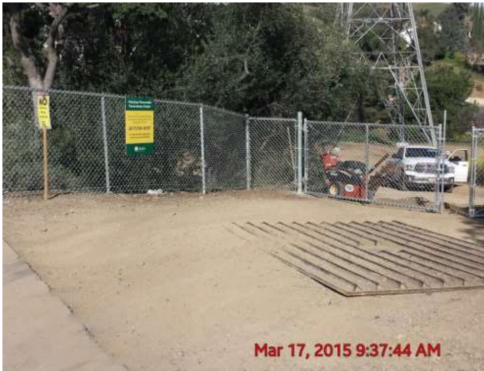
Figure 7: Equipment left in the nesting bird buffer after a one-hour hold was placed on the construction crew's activities at Tower M52-T1 (Segment 8, Phase 4) (photo courtesy of SCE).
