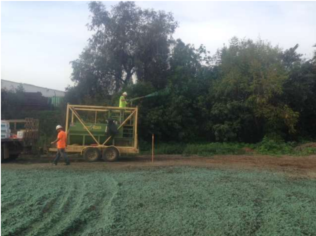
Figure 3: Hydroseeding at a wire site along Segment 8, Phase 4 (photo courtesy of SCE).
