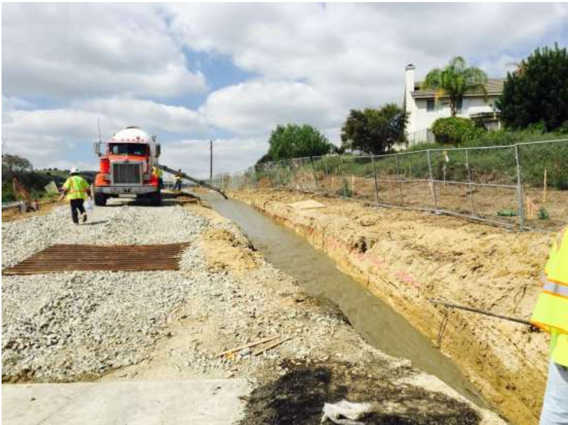
Figure 4: Backfilling the trench with concrete slurry mix between VC #9 and #10, 500 kV Underground.
