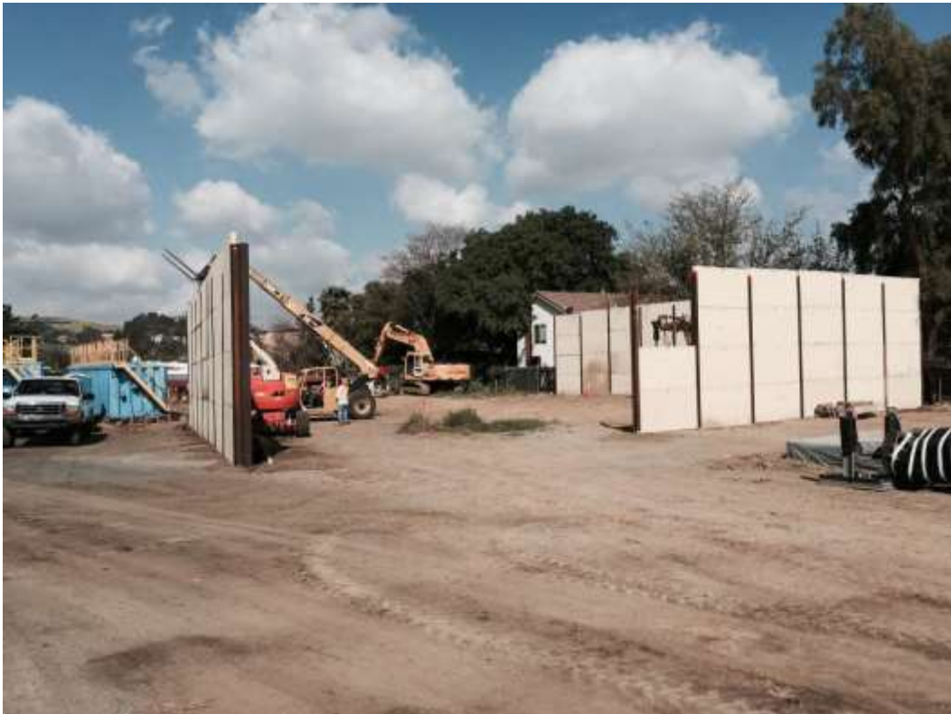
Figure 5: Installation of sound walls to accommodate HDD operations near VC #12, 500 kV Underground.
