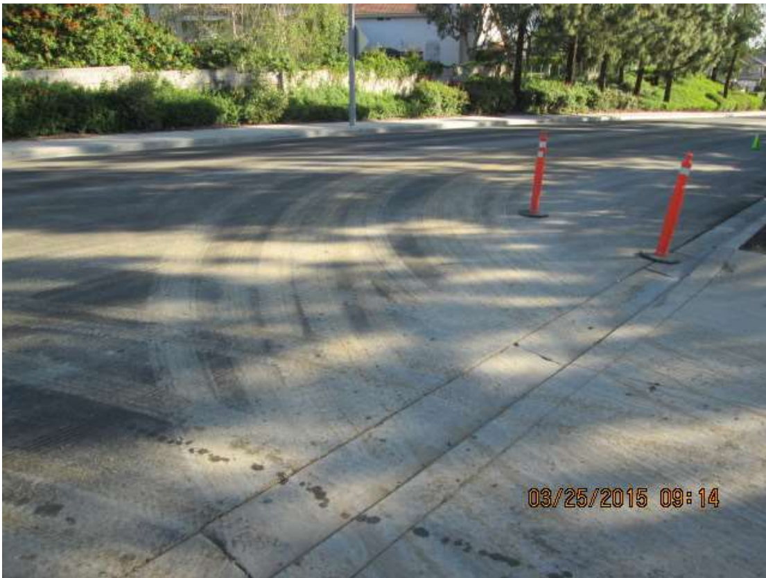
Figure 7: Excessive track-out at the WTS entrance reported by SCE Monitor, 500 kV Underground (photo courtesy of SCE).
