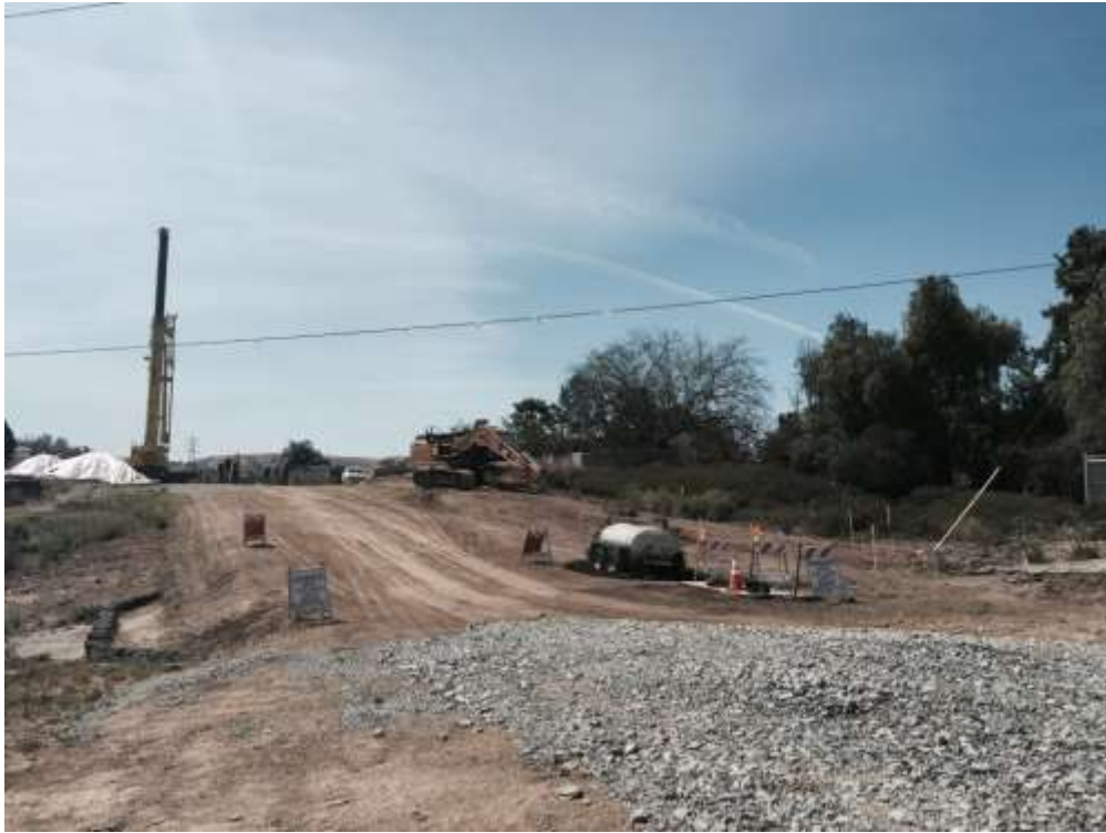
Figure 9: Telecommunication line that was struck at VC#9 which resulted in a Safety Stand Down, 500 kV Underground.
