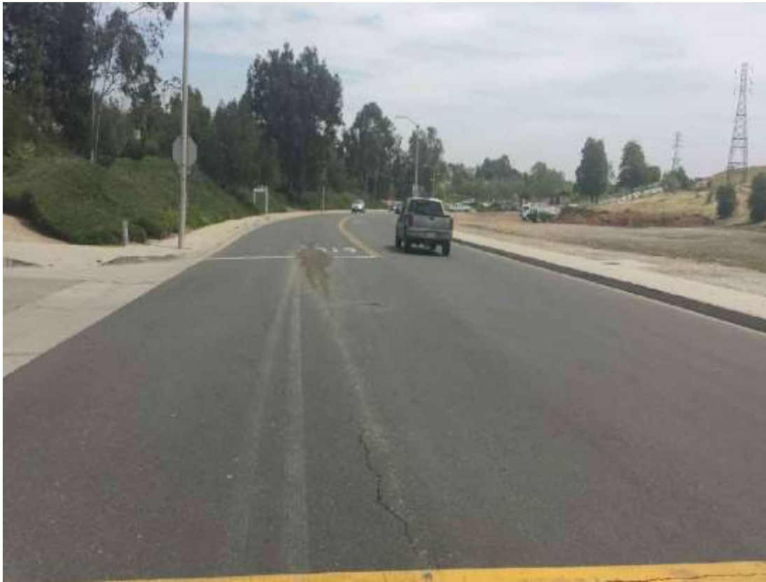
Figure 7: Concrete spill that occurred on Eucalyptus Ave, 500 kV Underground. (Photo Courtesy of SCE)
