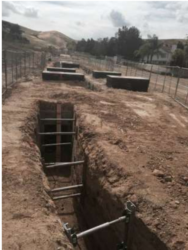
Figure 5: The CPUC EMs identified inadequate wildlife escape ramps installed in a trench near VC #5 which is approximately 10-12 feet deep. The ramps were too steep to allow any wildlife to escape and were replaced.
