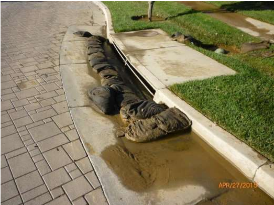
Figure 9: Post-storm offsite discharge observed flowing into storm drain along Canon Drive (photo courtesy of SCE).
