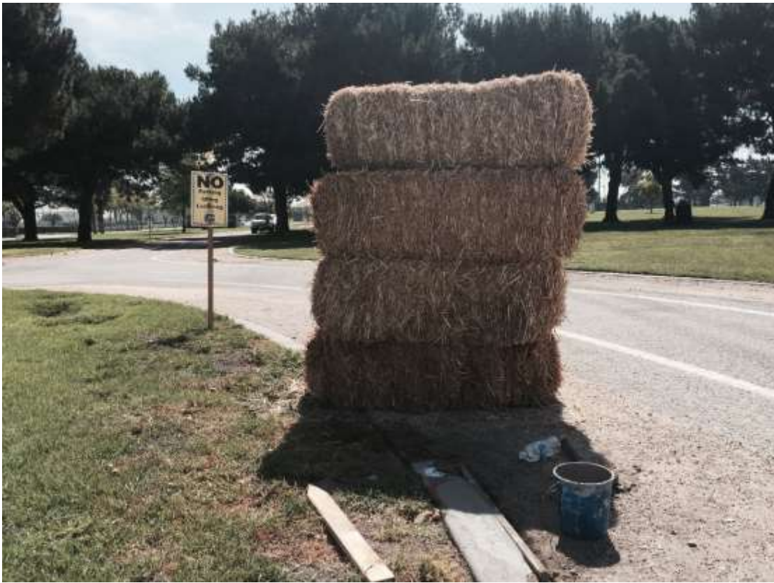
Figure 3: Concrete patchwork on the public walkway in Ayala Park (note hay bales as sound barrier for blackbird nesting colony).
