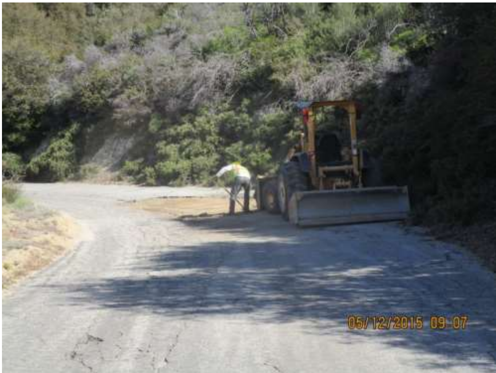
Figure 2: Road grading activities on Mt Gleason Road, Segment 11C (Photo courtesy of FRED).
