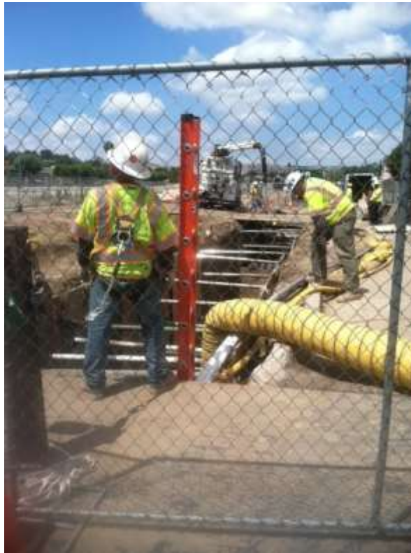
Figure 3: Conduit installation and backfill process along trenched area from VC#14 to Pipeline Avenue, 500 kV Underground.
