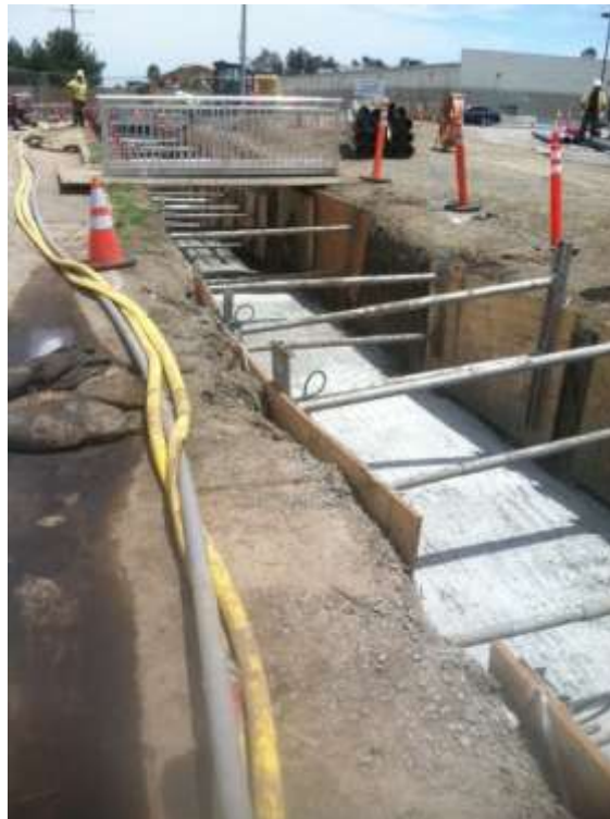
Figure 4: Conduit installation and backfill process along trenched area from VC#14 to Pipeline Avenue, 500 kV Underground.
