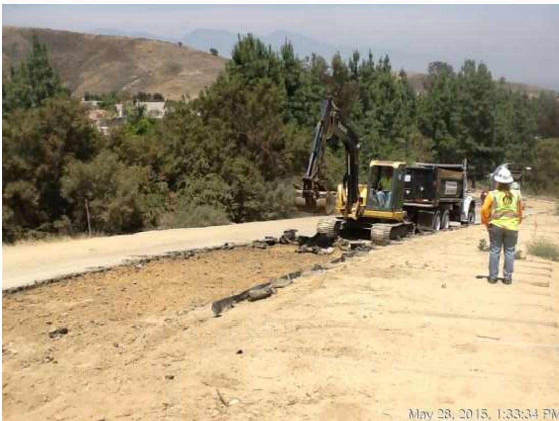
Figure 6: Asphalt removal for Class II Base preparation for driveway to WTS, 500 kV underground.
