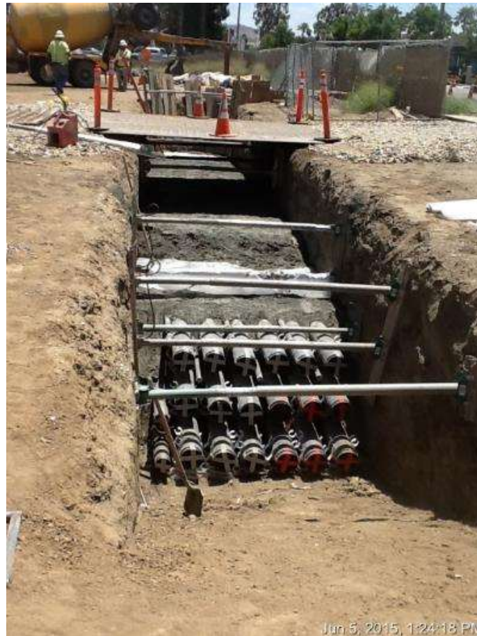
Figure 6: Conduit installation and backfilling trenchline across Pipeline Avenue into the ETS, 500 kV underground.
