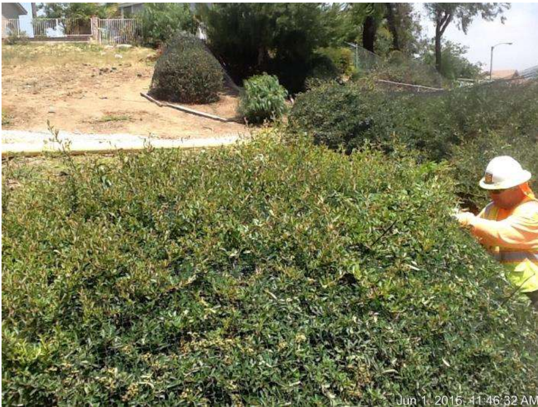
Figure 3: Vegetation trimming occurring on vegetation growth through bird exclusion netting at VC #11, 500 kV Underground.
