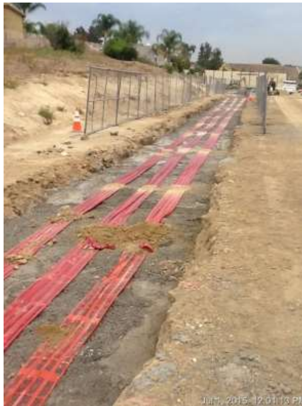
Figure 3: Preparing concrete-filled trenchline between VC #10 and VC #11 for soil backfilling activities, 500 kV Underground.
