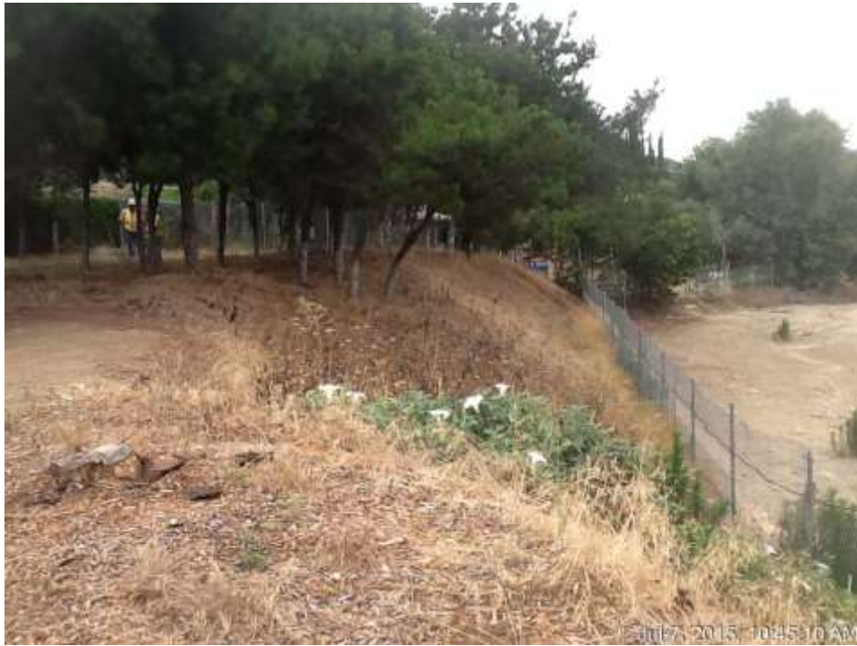
Figure 3: Fence installation along the edge of the right-of-way west of VC #12, 500 kV Underground.
